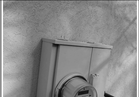
Lack of sealant
