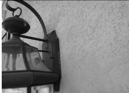
Lack of sealant
