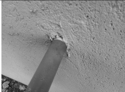
Lack of sealant
