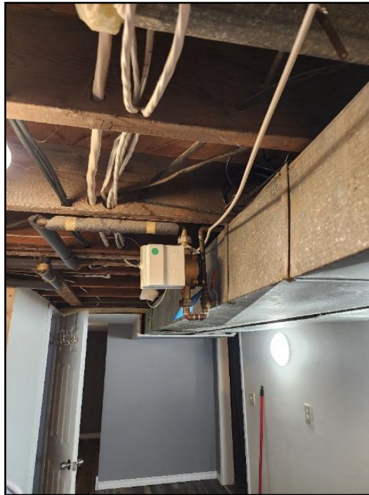
23. Main water shut off
