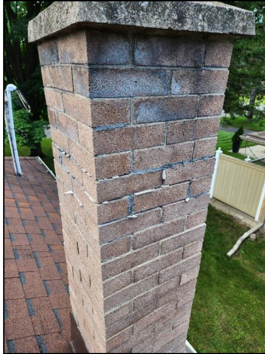
19. Loose, missing or deteriorated mortar
