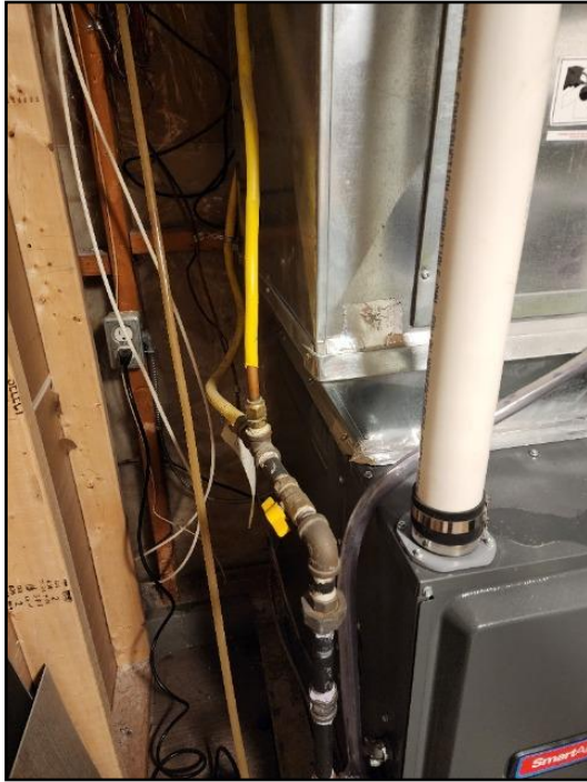
14. Main fuel shut off
