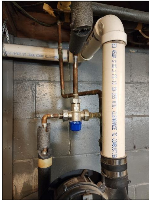
22. Tempering/mixing valve installed
