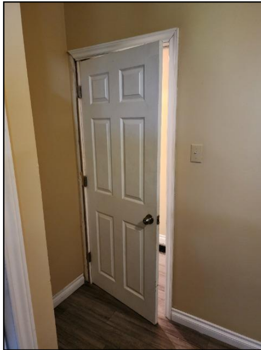
27. Loose or poor fit
