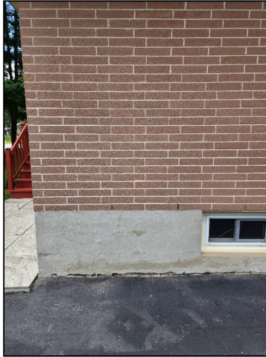
5. Typical minor cracks
