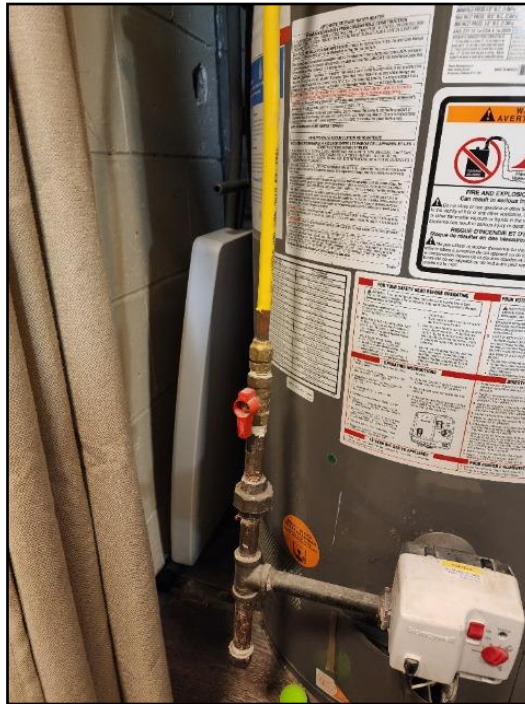
25. Main fuel shut off
