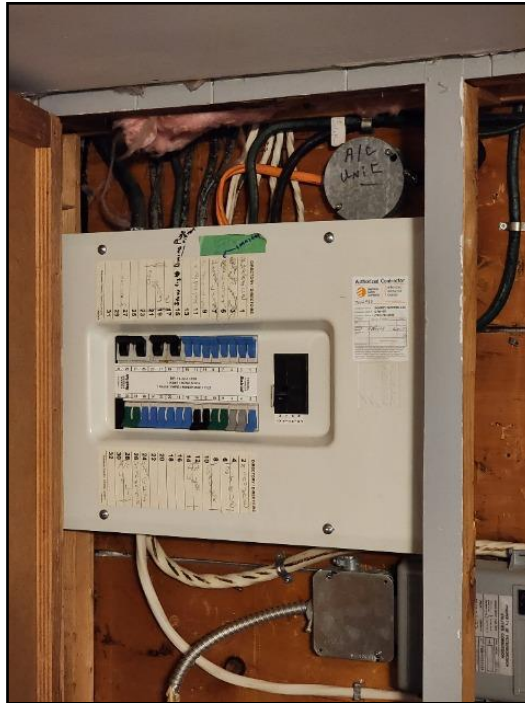
6. Main electrical disconnect
