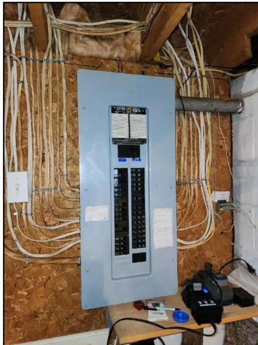
8. Main electrical disconnect
