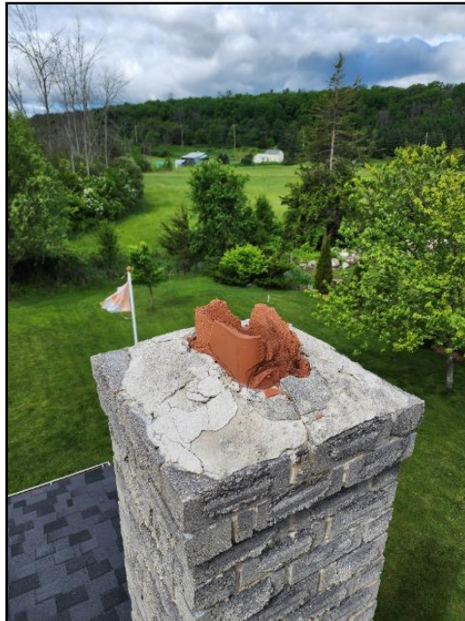
16. Cracked or damaged
