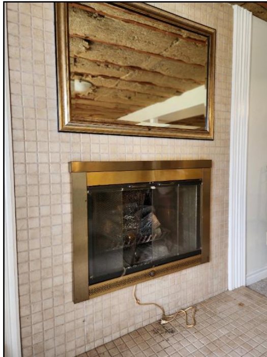
13. Wood-burning fireplace - not in service
