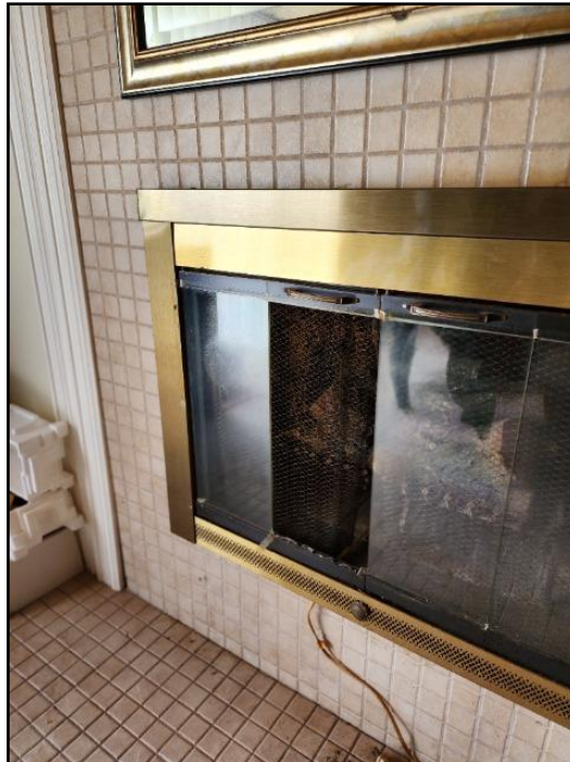
17. Cracked or broken glass
