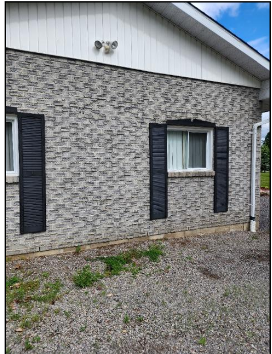
5. Typical minor cracks
