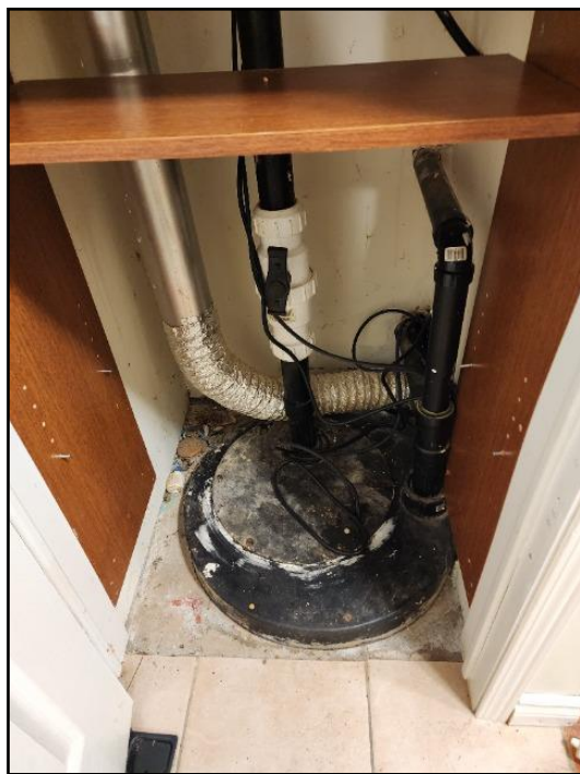
21. Solid waste pump (ejector pump)
