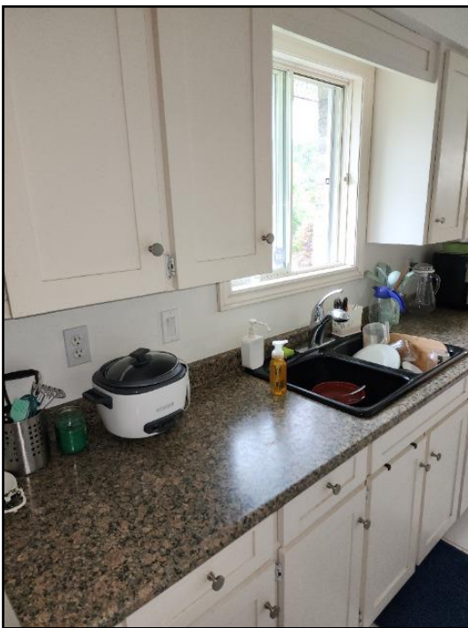
11. No GFCI/GFI (Ground Fault Circuit...
