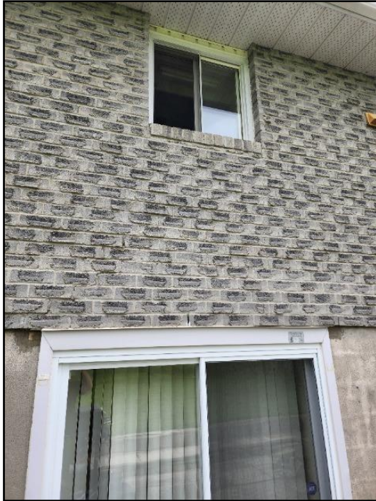
6. Typical minor cracks
