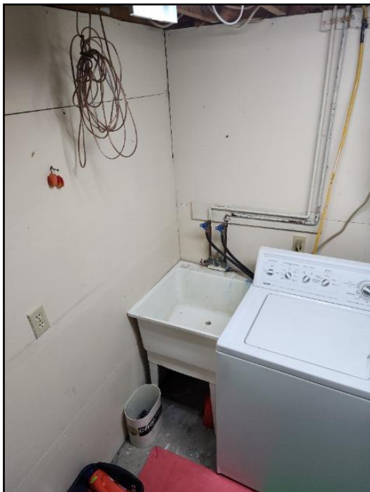
10. No GFCI/GFI (Ground Fault Circuit...
