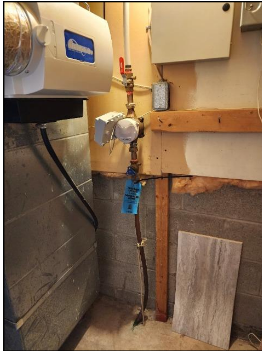
27. Main water shut off
