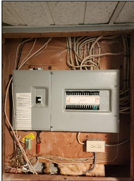
6. Main electrical disconnect
