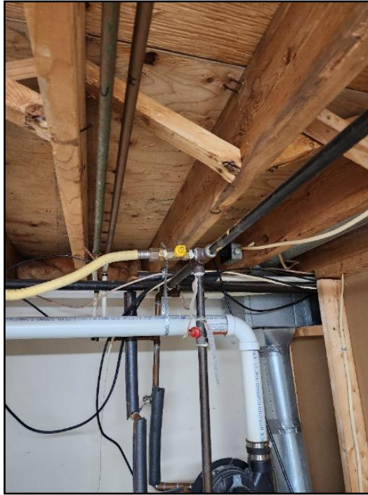
29. Main fuel shut off
