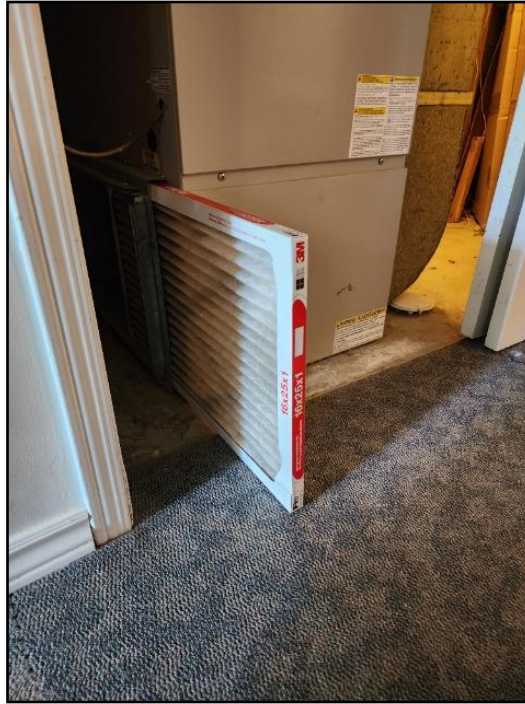
22. Replace - regular maintenance
