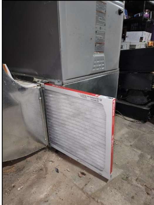
45. Replace - regular maintenance
