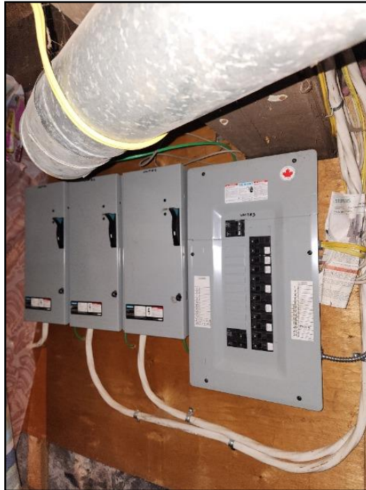
18. Main electrical disconnects
