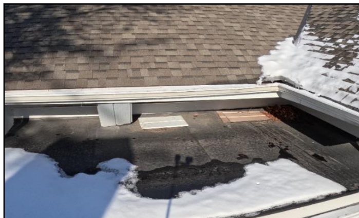
5. Loose or missing pieces
