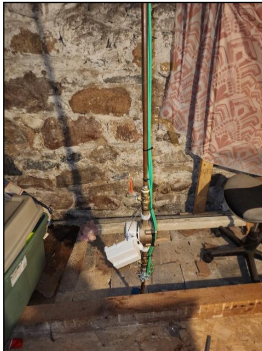
47. Main water shut off
