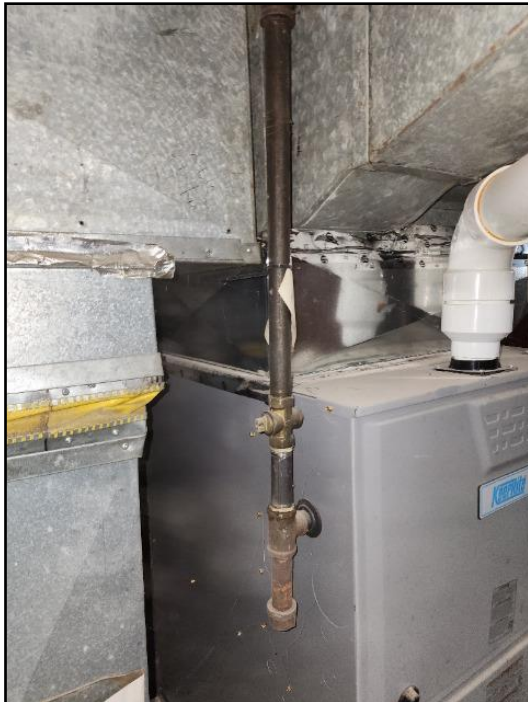
37. Main fuel shut off
