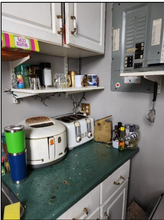
30. No GFCI/GFI (Ground Fault Circuit...
