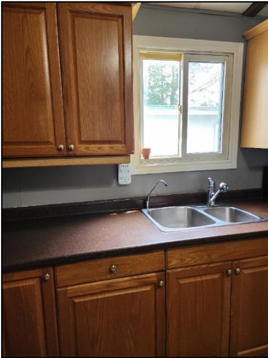
13. No GFCI/GFI (Ground Fault Circuit...
