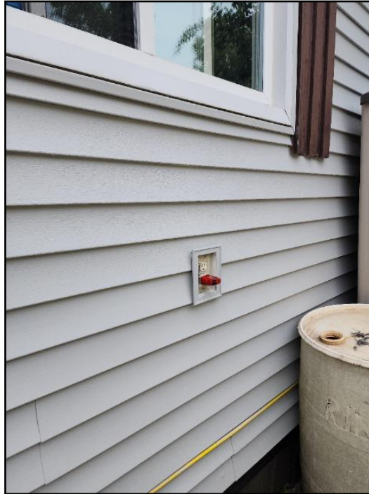
14. No GFCI/GFI (Ground Fault Circuit...
