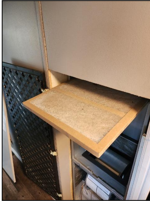
17. Replace - regular maintenance
