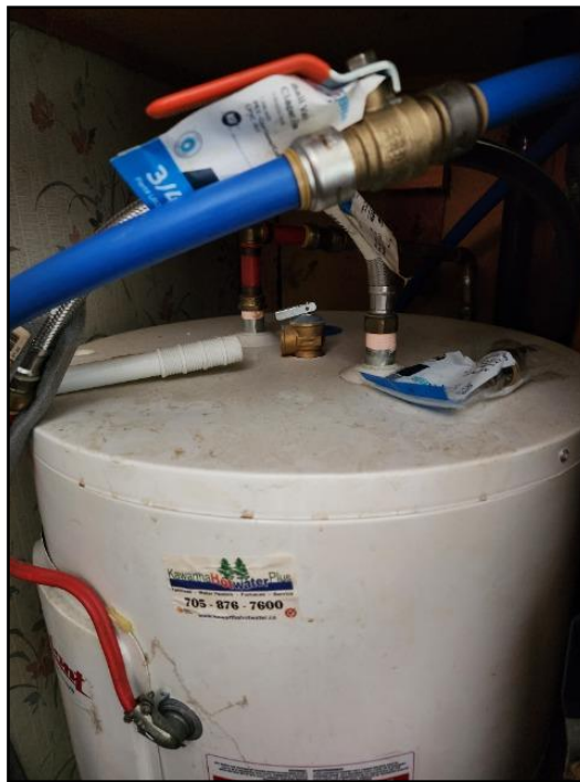
22. Discharge tube disconnected
