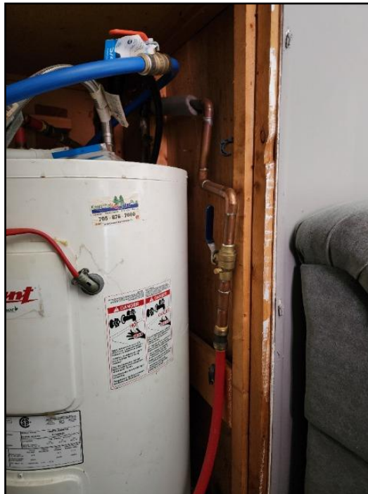
19. Main water shut off
