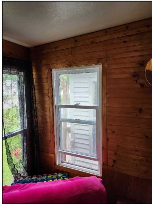
23. Lost seal on double glazing
