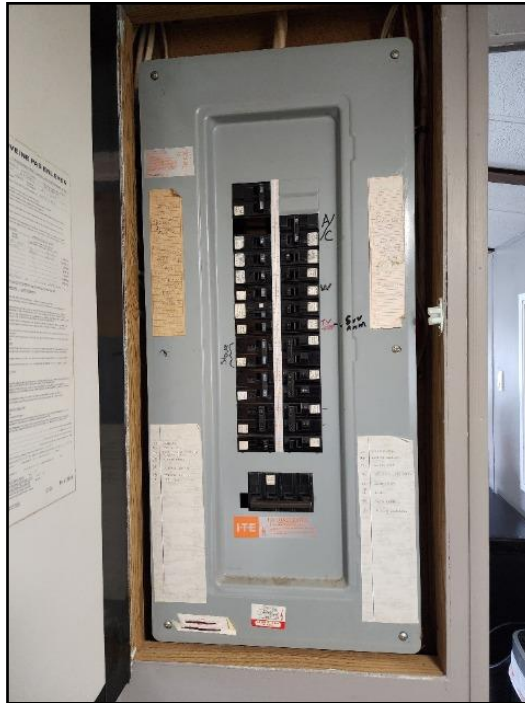
9. Main electrical disconnect
