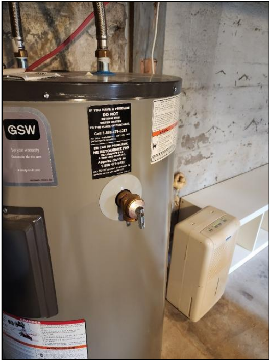
26. Discharge tube missing
