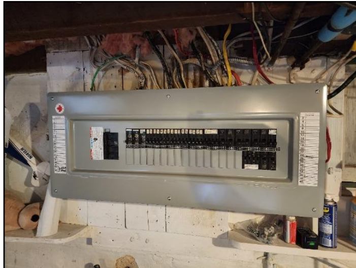
9. Main electrical disconnect
