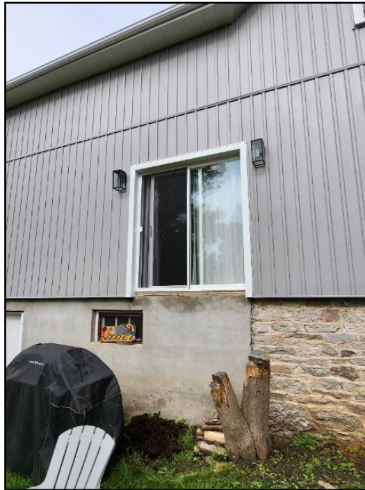
5. Stairs and landing missing
