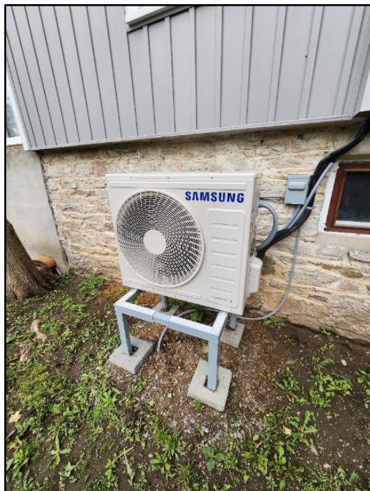
21. Ductless (Mini split) system
