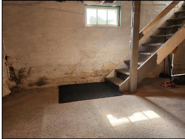
28. Crumbling/spalling masonry, concrete or...
