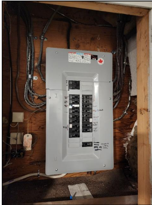
3. Main electrical disconnect
