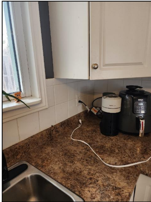
9. No GFCI/GFI (Ground Fault Circuit...
