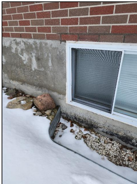
1. Typical minor cracks
