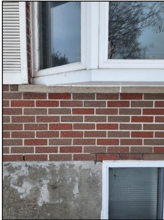
2. Typical minor cracks
