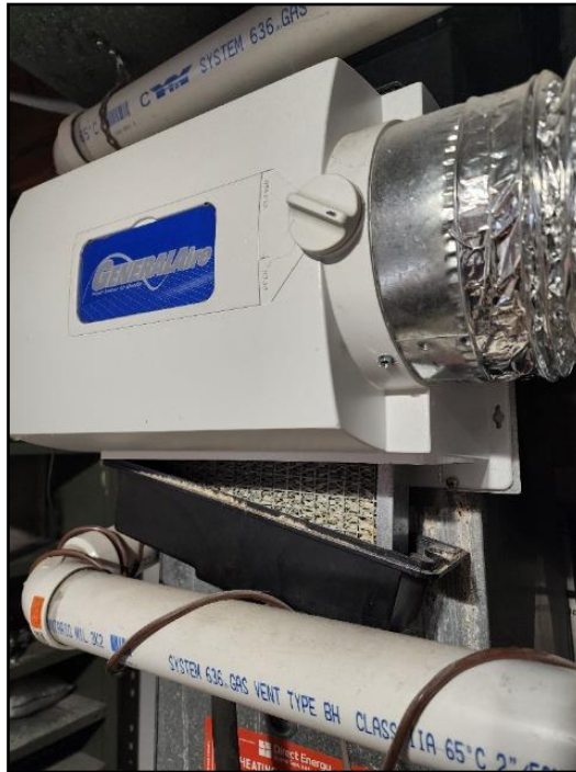
18. Clean pad/mesh - regular maintenance
