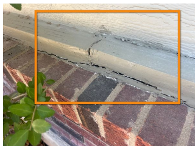
Caulk and seal needed - multiple locations
