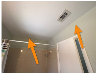
Ceiling Sheetrock cracks - hall bathroom
