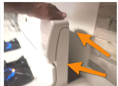
Missing anti tip device - stove
