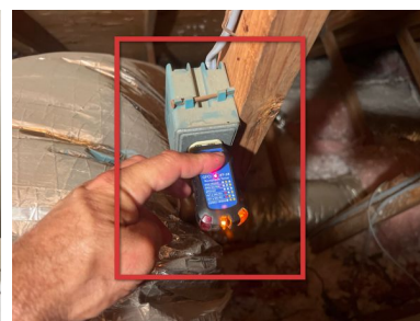
GFCI missing in attic
