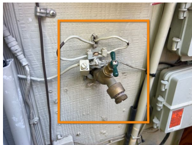
PEX line present - Could not verify bonding at left exterior hose bib
