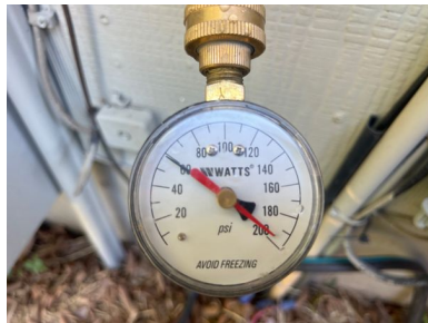
Static water pressure approximately 58 psi
