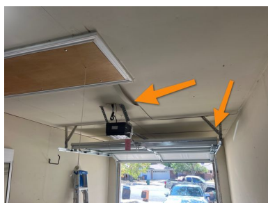
Peeling tape joints - garage ceiling
