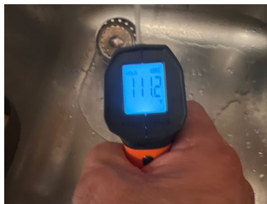
111° average hot water at all faucets
