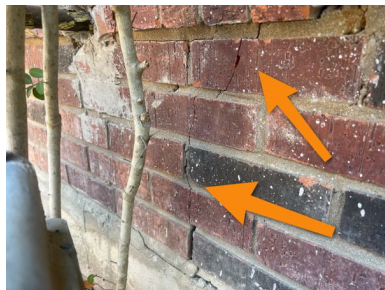
Left exterior brick/mortar crack at exterior wall
