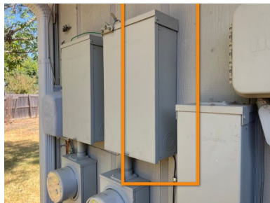
Caulk and seal needed - electrical panels - left exterior wall
