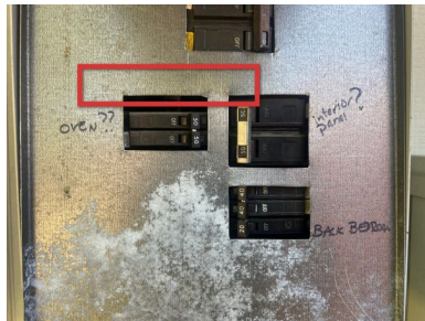
Open breaker slot - main panel
