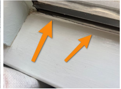
Caulk and seal needed at multiple interior windows
