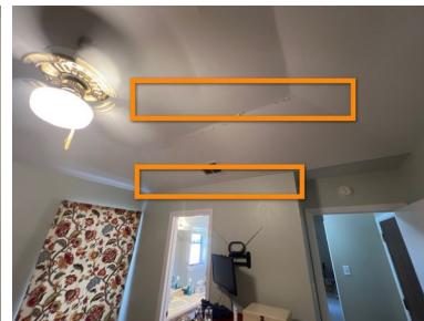
Ceiling Sheetrock cracks - master bedroom
