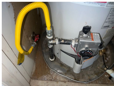
Garage water heater unit
