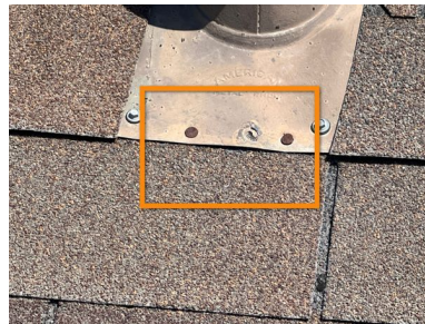
Exposed nail heads at multiple locations throughout rooftop
