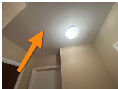
Ceiling Sheetrock crack - garage hallway
