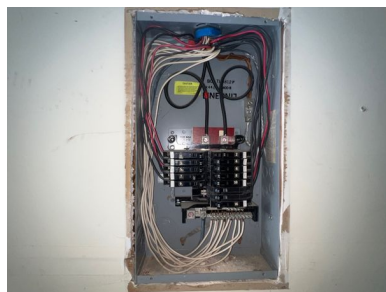
Sub panel - no AFCIs present - garage
