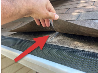
Starter course improporly installed at roof perimeter
