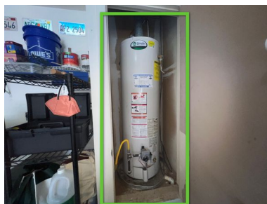
Garage water heater unit
