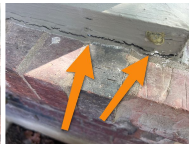
Caulk and seal needed - multiple locations
