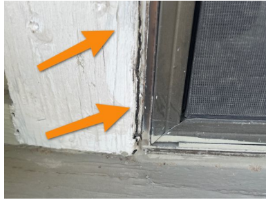
Caulk and seal needed - multiple exterior windows
