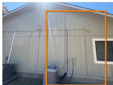
Caulk and seal needed - multiple locations
