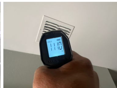
111° average heat at interior registers
