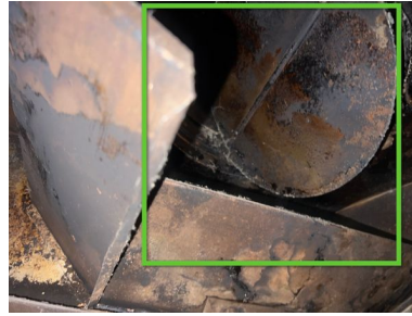
Fireplace dampner - Working as Intended
