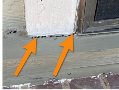
Caulk and seal needed - multiple exterior windows
