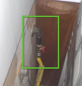
Gas shut off valve - behind stove
