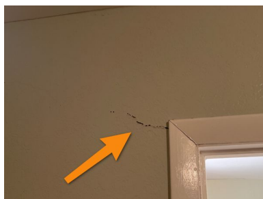
Sheetrock crack - master bedroom
