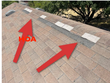
Loose/ torn shingles - roof ridge
