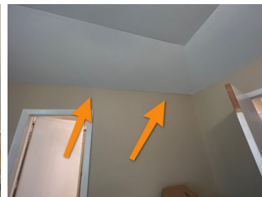
Ceiling Sheetrock cracks - guest bedroom
