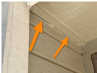
Caulk and seal needed - multiple locations
