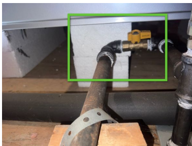
Gas shut off valve - attic furnace unit
