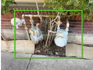
Gas meter - left exterior wall
