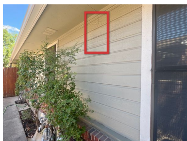
Damaged lap siding - left exterior wall
