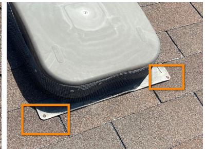
Exposed nail heads at multiple locations throughout rooftop
