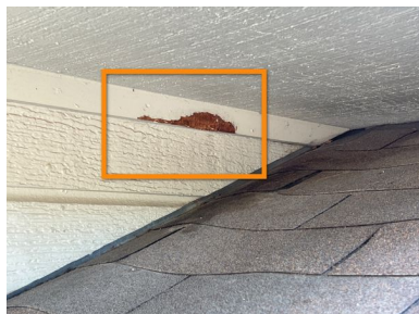
Rodent damage at frieze boards - front roof
