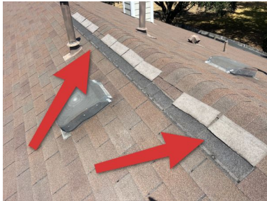
Loose torn shingles - roof ridge
