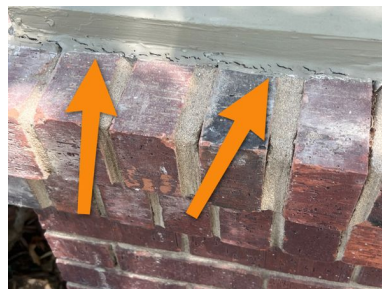
Caulk and seal needed - multiple locations
