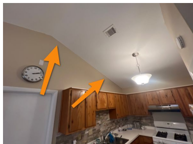
Ceiling Sheetrock cracks - draining room
