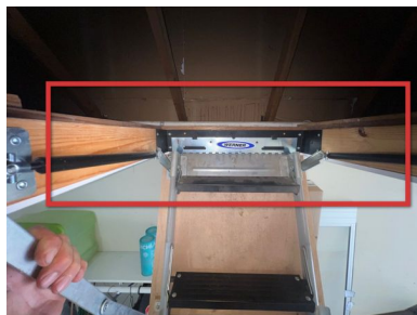
Missing 16D nails at attic ladder assembly - garage
