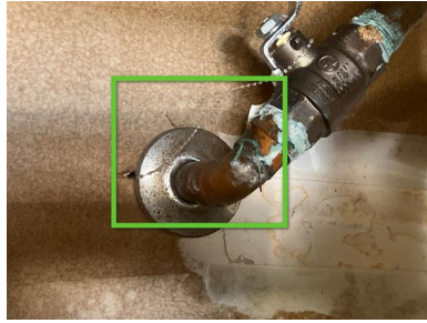
Copper water lines visible - garage
