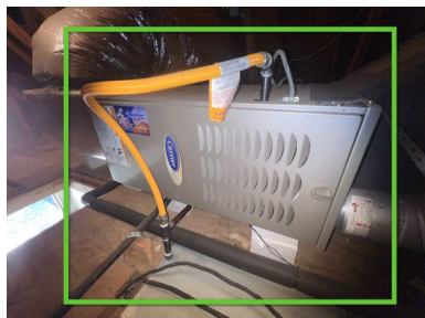
Attic furnace unit
