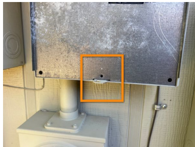
Missing screw at dead front - main panel
