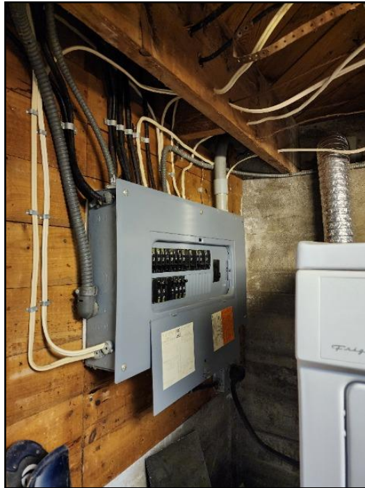
8. Main electrical disconnect
