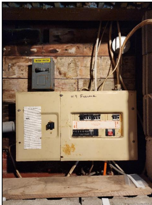
9. Main electrical disconnect
