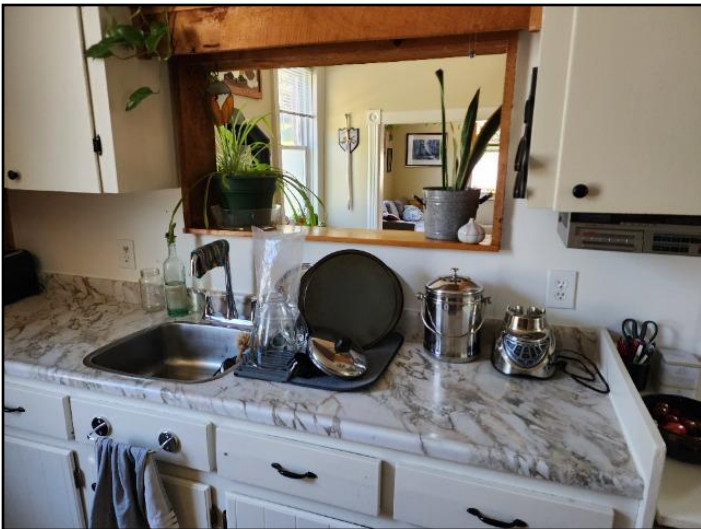
21. No GFCI/GFI (Ground Fault Circuit...
