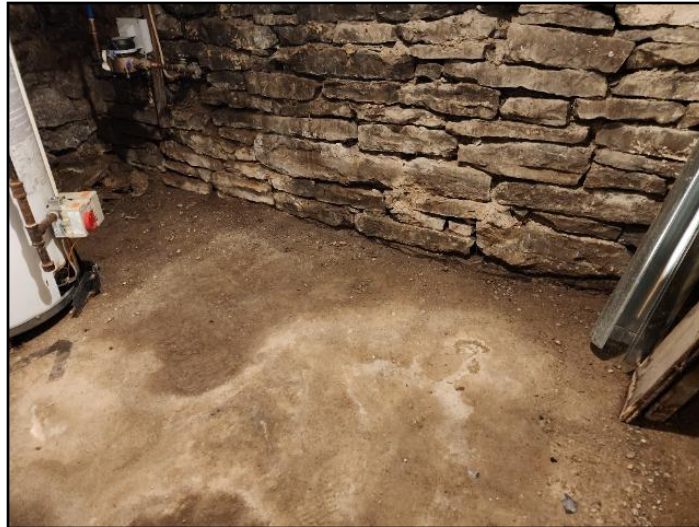
41. Dampness on floor or walls
