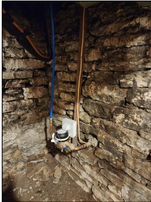
32. Main water shutn off
