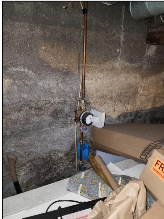
26. Main water shut off
