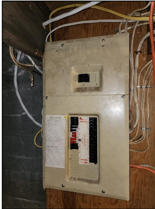
12. Main electrical disconnect
