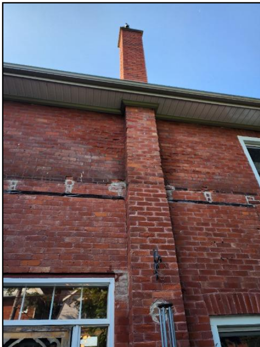
9. Masonry deteriorated or spalling
