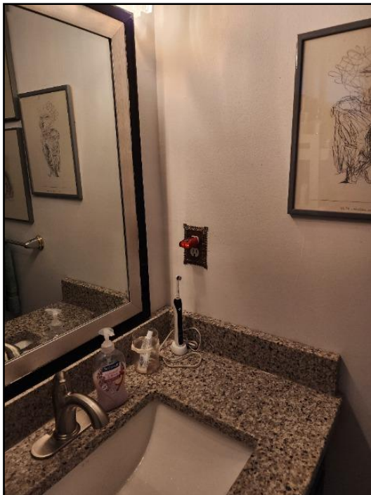
16. No GFCI/GFI (Ground Fault Circuit...
