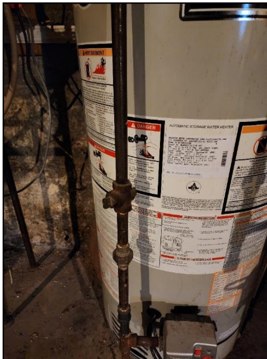
28. Main fuel shut off
