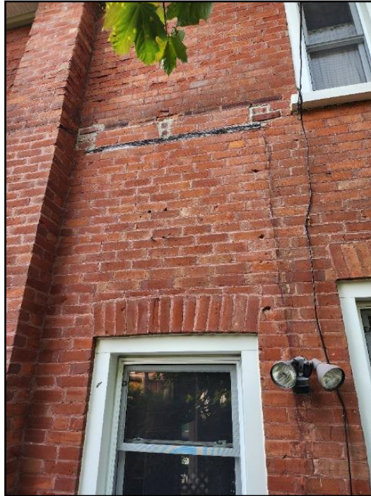
11. Typical minor cracking
