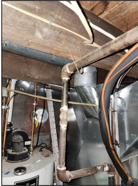
19. Main fuel shut off
