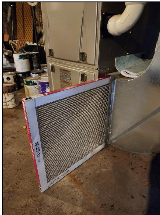
22. Replace - regular maintenance
