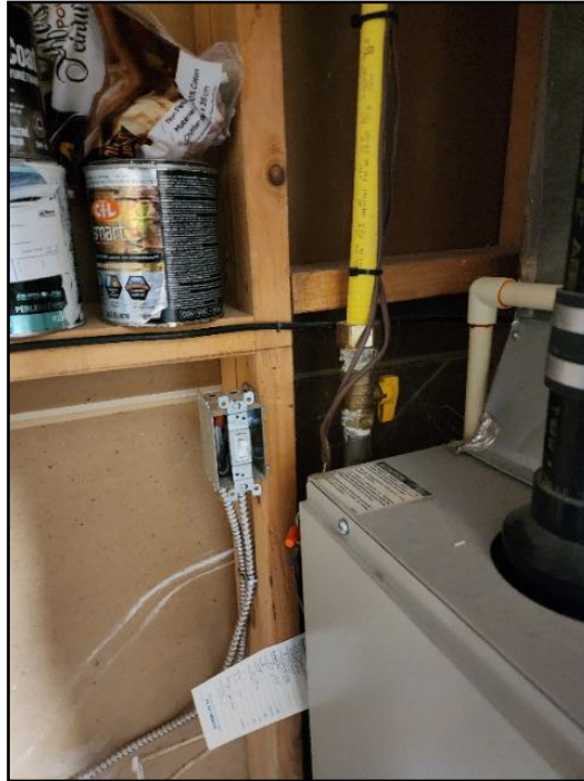
11. Main fuel shut off & electrical disconnect
