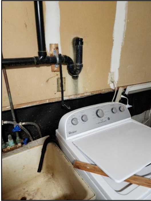
8. No GFCI/GFI (Ground Fault Circuit...
