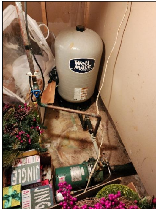
20. Well pump & pressure tank
