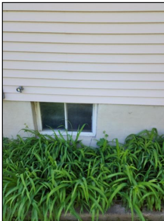
5. Typical minor cracks
