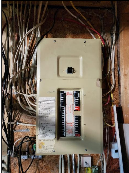
6. Main electrical disconnect
