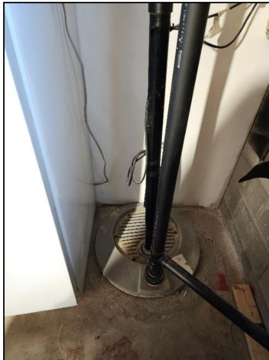
24. Solid waste pump (ejector pump)
