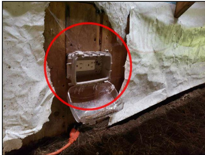
GFCI/GFI needed (Ground Fault Circuit...
