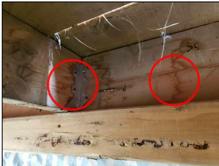
Missing Lag Bolts
