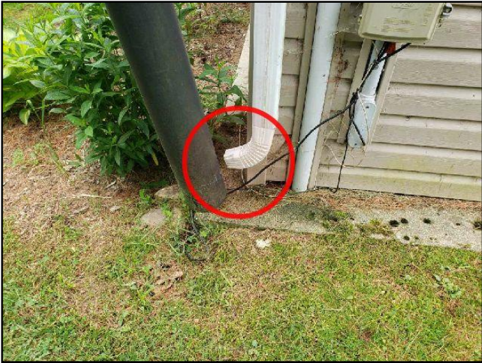
Discharge too close to building
