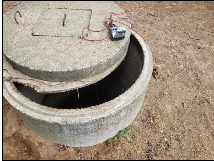
Lid Missing, Damaged.
