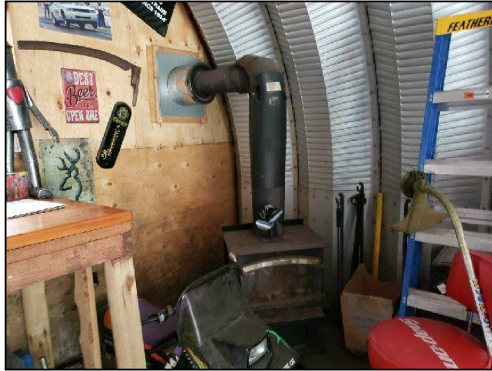
WETT Inspection Not performed
