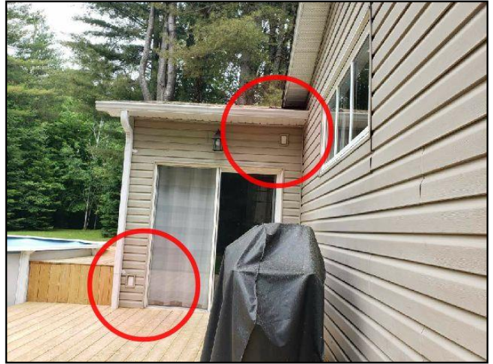
GFCI/GFI needed (Ground Fault Circuit...
