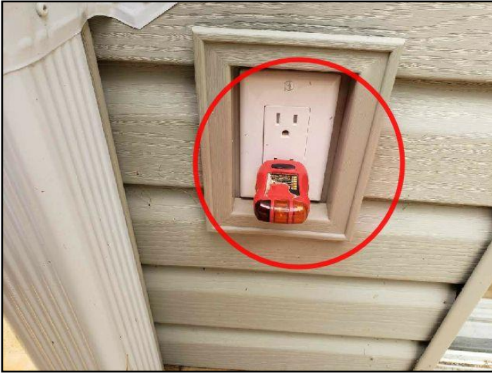
GFCI/GFI needed (Ground Fault Circuit...
