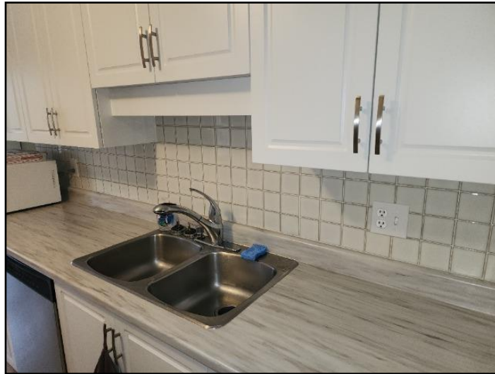
3. No GFCI/GFI (Ground Fault Circuit...
