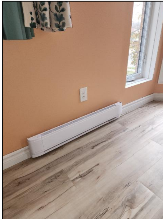
4. Electrical receptacle above heater
