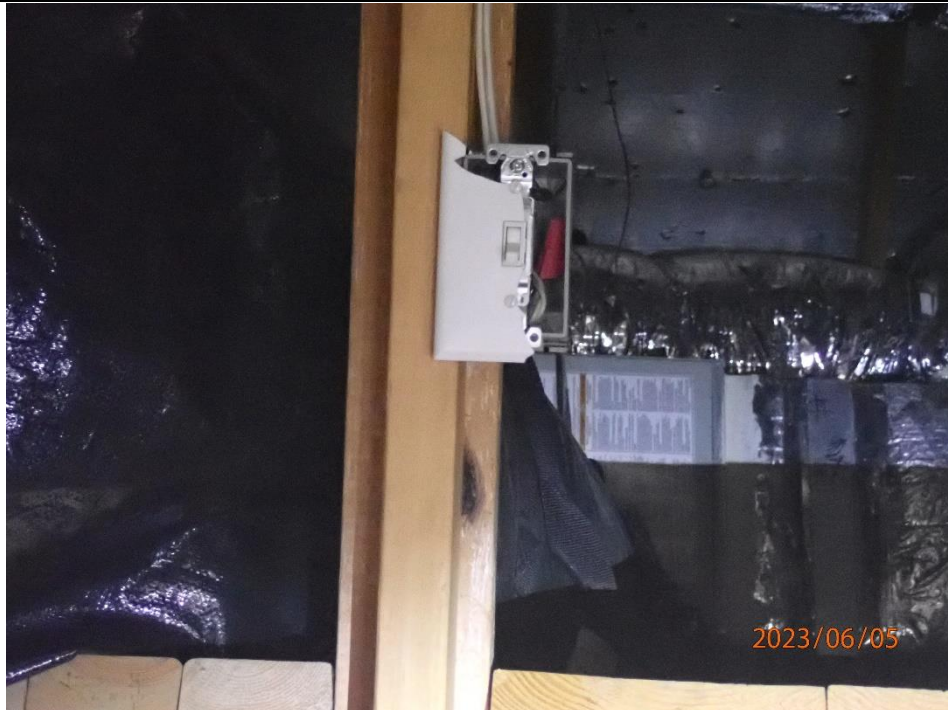
DAMAGED ELECTRICAL SWITCH COVER IN THE ATTIC
