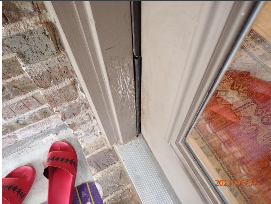
PET DAMAGE ON PATIO DOOR
