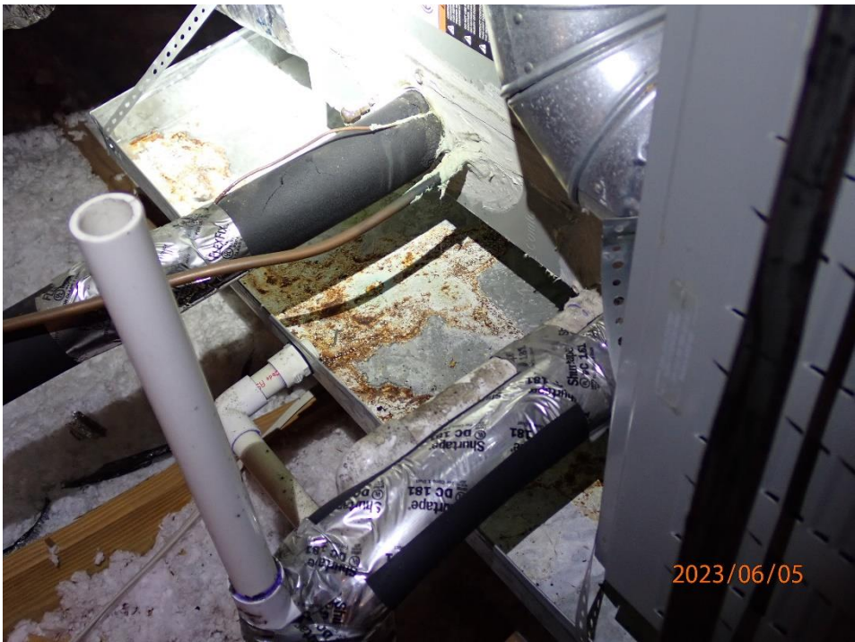
RUST IN A/C SECONDARY DRAIN PAN
