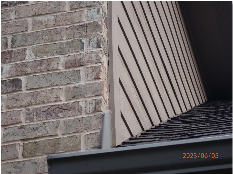
VERTICAL TRIM NEEDS TOUCH UP CAULK TO THE BRICK
