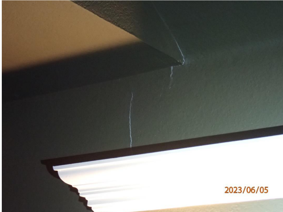
SETTLEMENT CRACKS IN WALLS AND CEILING
