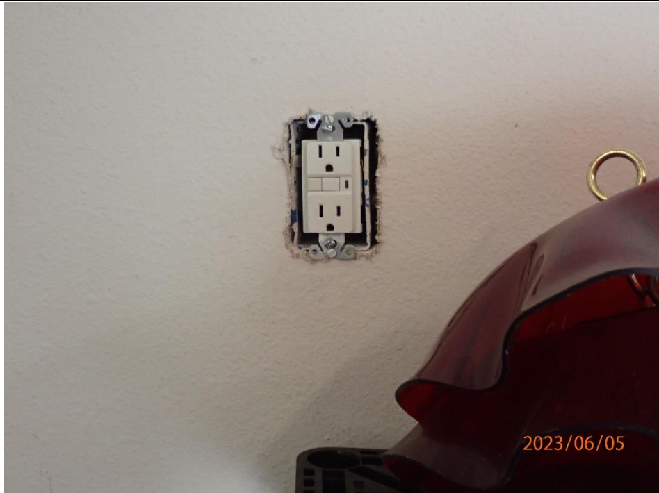
MISSING OUTLET COVER IN THE GARAGE
