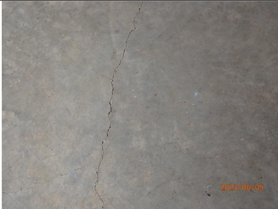
SETTLEMENT CRACKS IN THE GARAGE FLOOR
