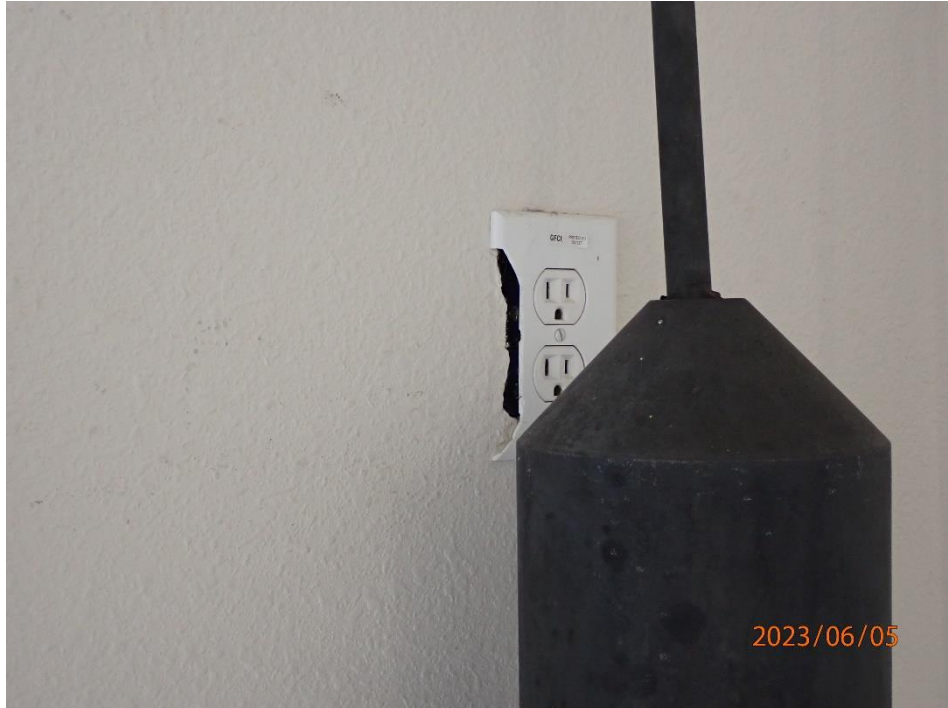
DAMAGED OUTLET COVER IN THE GARAGE
