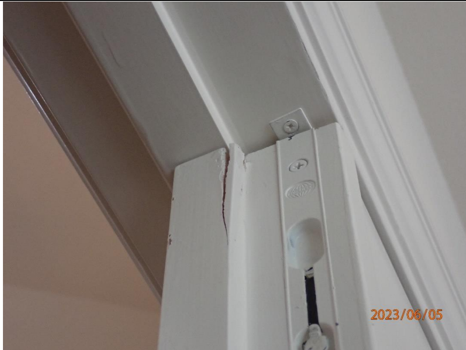
DAMAGED OFFICE DOOR EDGE
