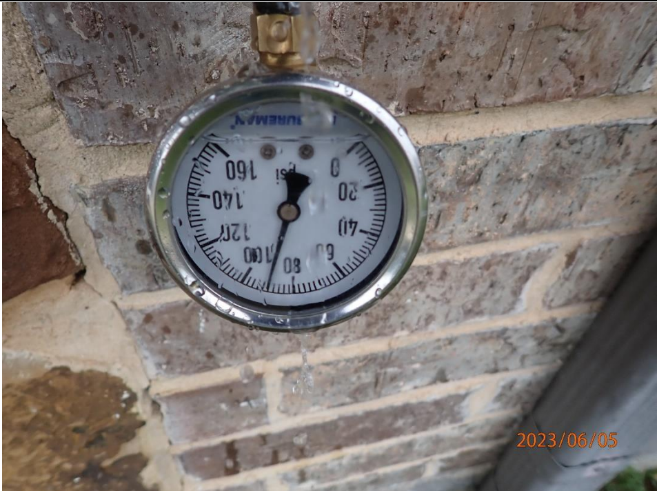
WATER PRESSURE WAS ABOVE 80 PSI AT THE TIME OF THE INSPECTION
