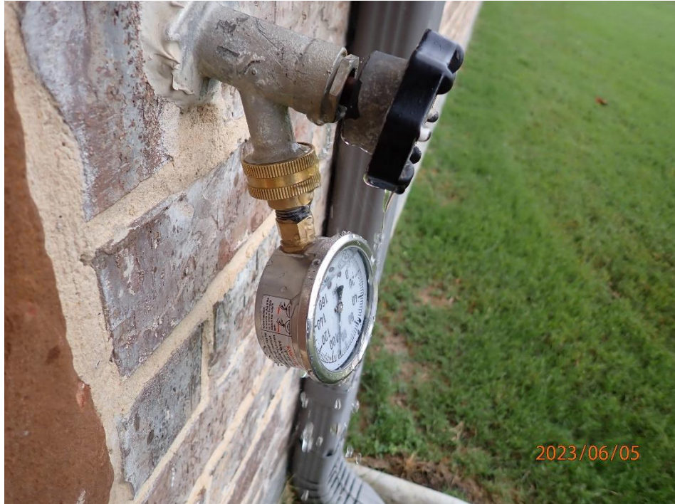
LEAK AT HOSE BIB WHEN IN USE
