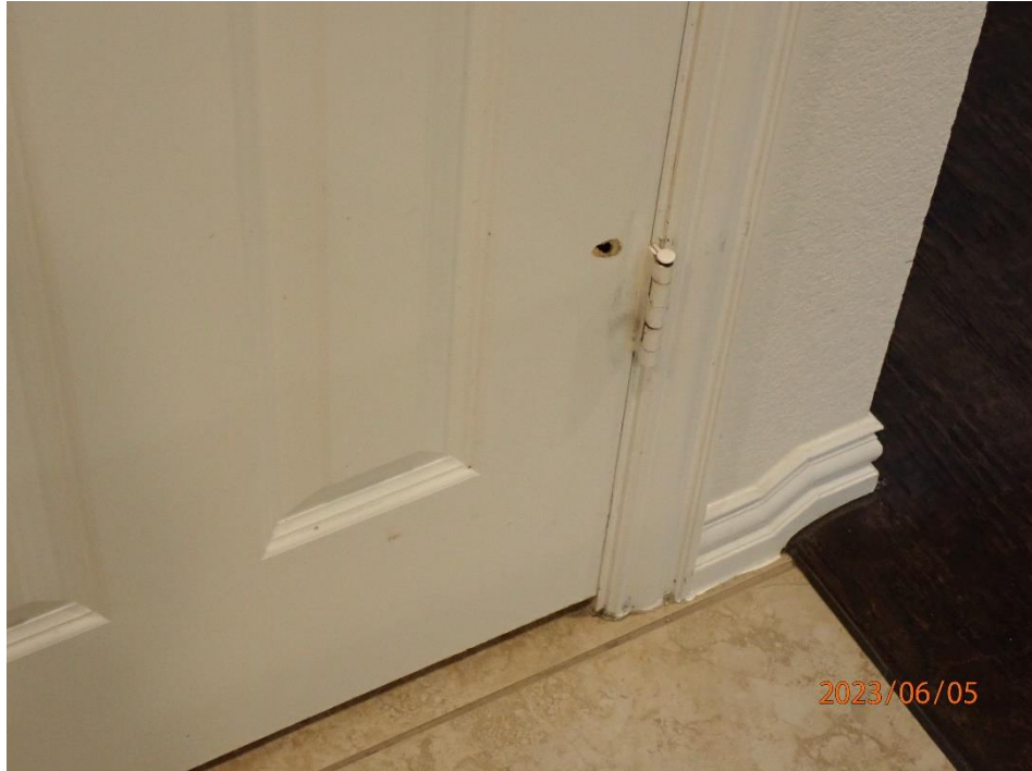
DAMAGED PANTRY DOOR
