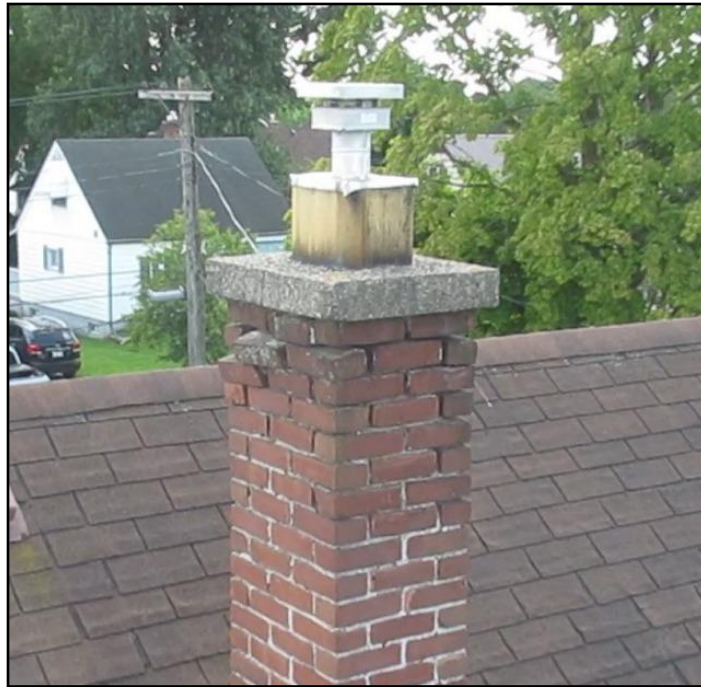
22. Loose, missing or deteriorated masonry
