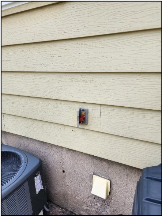
13. Test faulty on GFCI/GFI (Ground Fault...
