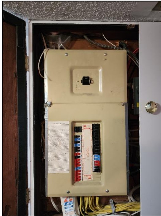
5. Main electrical disconnect
