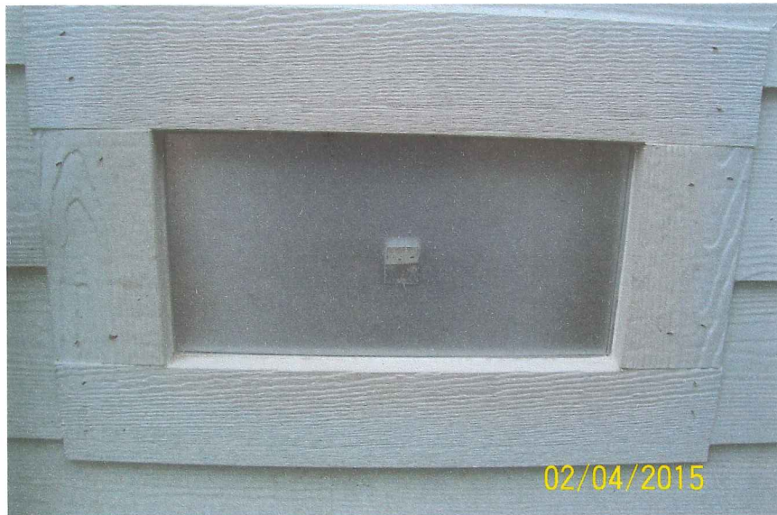
Typical engineered flood vent. See attached
