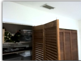
One or more of the closet doors have separations in the doors.
