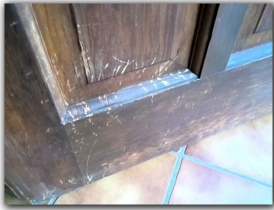
Surface damage was noted on the doors in various areas.
