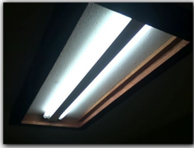
The utility room light fixture cover is missing.
