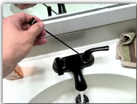
The drain stops were missing or did not work properly on one or more faucets.
