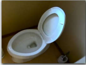
The master bathroom toilet is damaged and not functional at the time of inspection.
