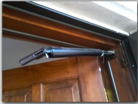
The front storm door hardware is detached.
