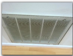
The filter is over a year old and in need of replacement.
