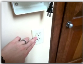
Loose mounted receptacles were observed in one or more areas.
