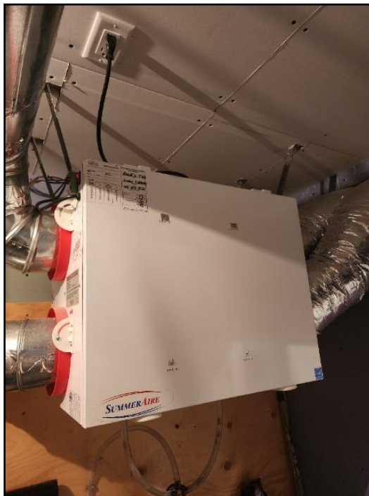
12. Heat recovery ventilator (HRV)
