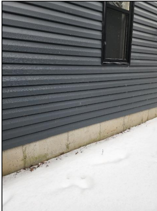
1. Typical minor cracks
