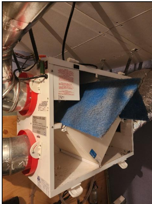
14. Clean filters - regular maintenance
