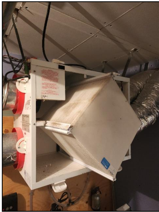
13. Clean core - regular maintenance
