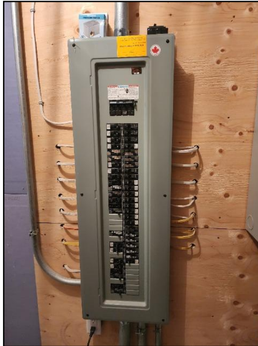
2. Main electrical disconnect
