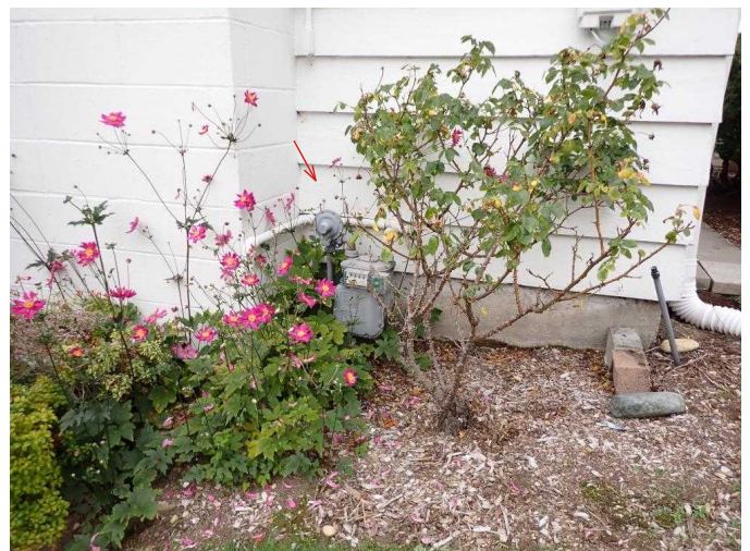
#6 Gas meter located on E side of house.
