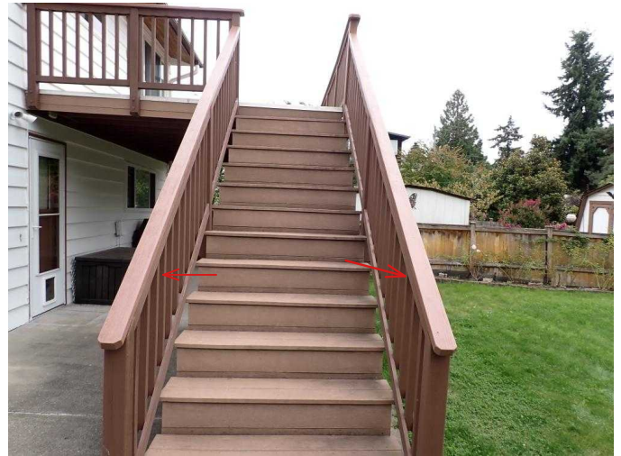
#14 Railings on deck access steps are loose on install.
