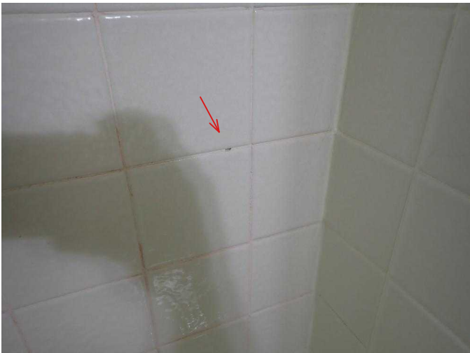
#45 Small sections of grout missing from lower level bath surround, water intrusion spots, need to be sealed.
