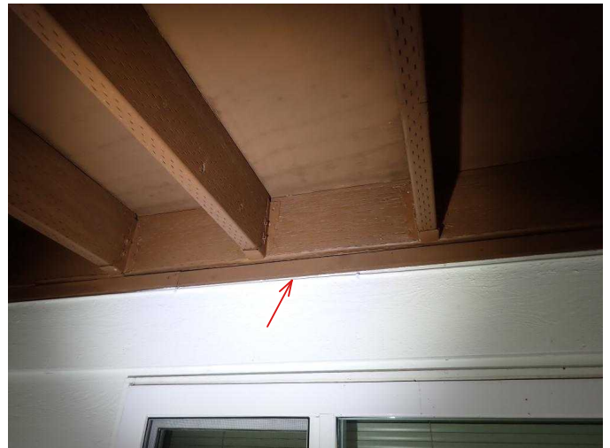
#10 Deck is not bolted to house (safety).
