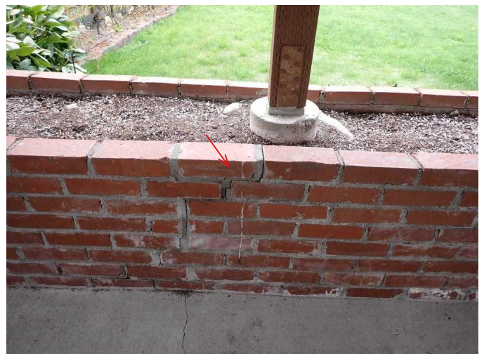
#12 Moderate staggered settling crack in patio flower bed.
