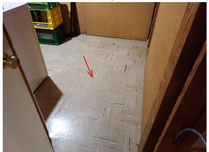
#48 Test linoleum tile for asbestos prior to working with, altering or removing linoleum tile.
