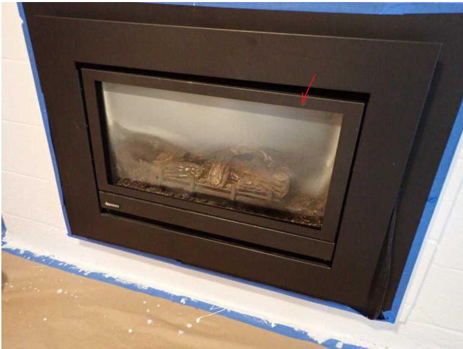
#43 Glass needs cleaning, only use fireplace glass cleaner.
