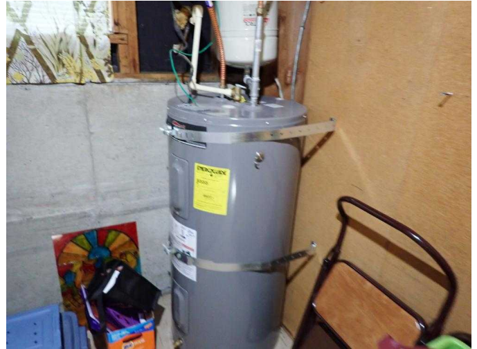
#50 Water heater located in laundry room.
