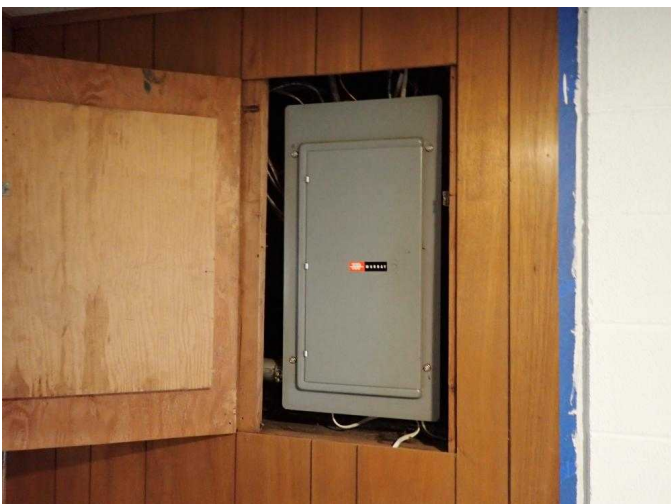
#53 Electric panel located in family room.
