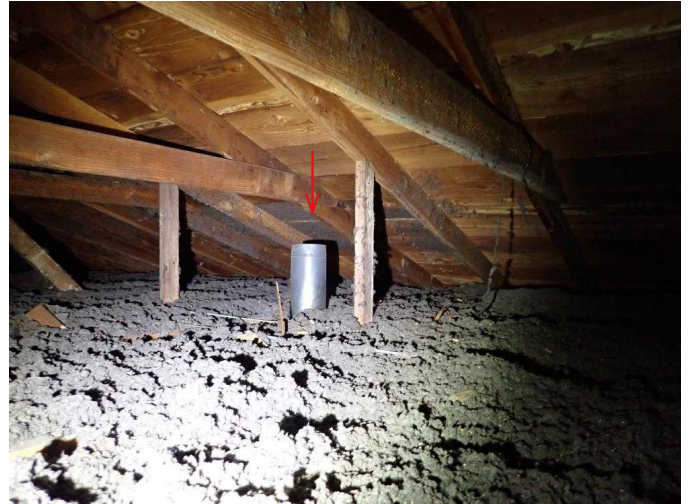
#38 Kitchen fan vents directly into attic, needs to be sealed transition to exterior.
