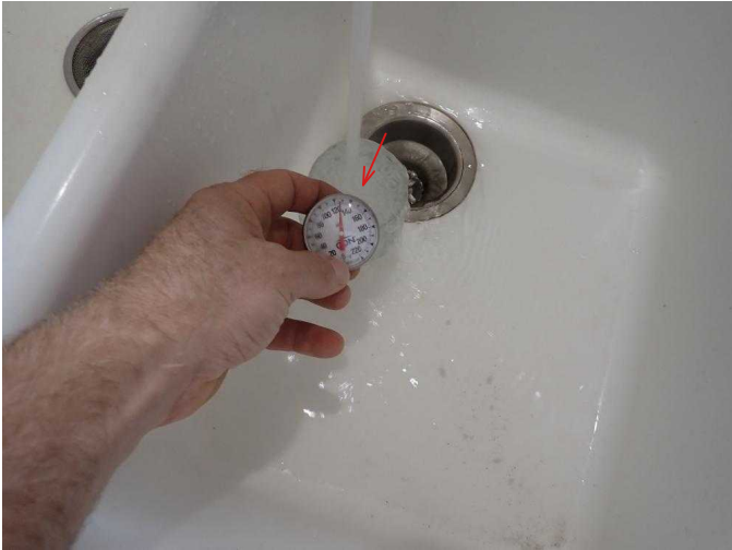
#31 Water temperature is 130 deg F, should be lowered to 120 deg F to reduce the risk of scalding.
