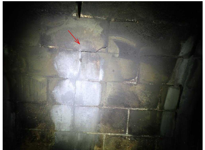
#28 Minor cracks in firebrick in back of living room firebox, needs to be sealed prior to use.
