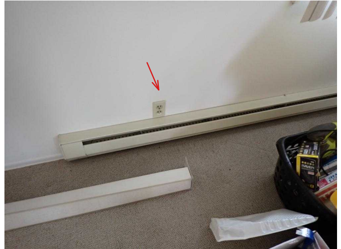
#26 Outlets over baseboard heaters need to be removed or relocated (safety).
