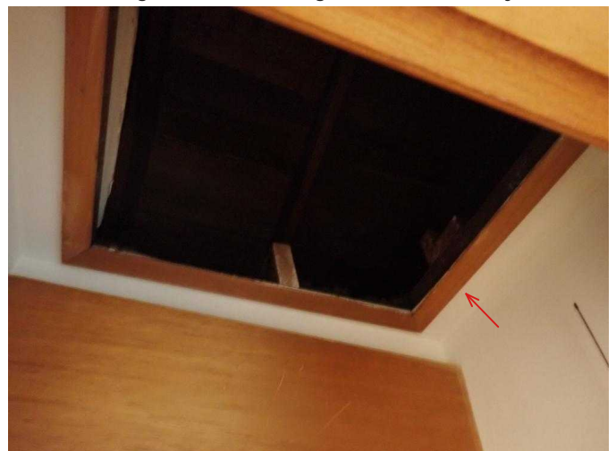
#36 No air seal present for attic access hatch. Access located in first floor hall closet.
