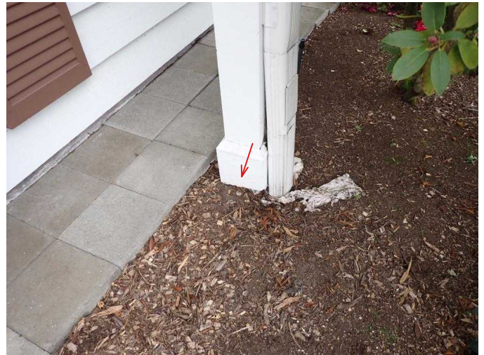
#2 W front porch roof support pillar is no longer attached to footing.
