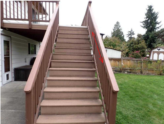
#13 No graspable handrails present for deck access steps (safety).
