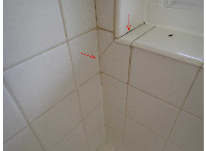
#32 Minor cracks in first floor bath surround grout at corner junctions, water intrusion spots, need to be sealed.
