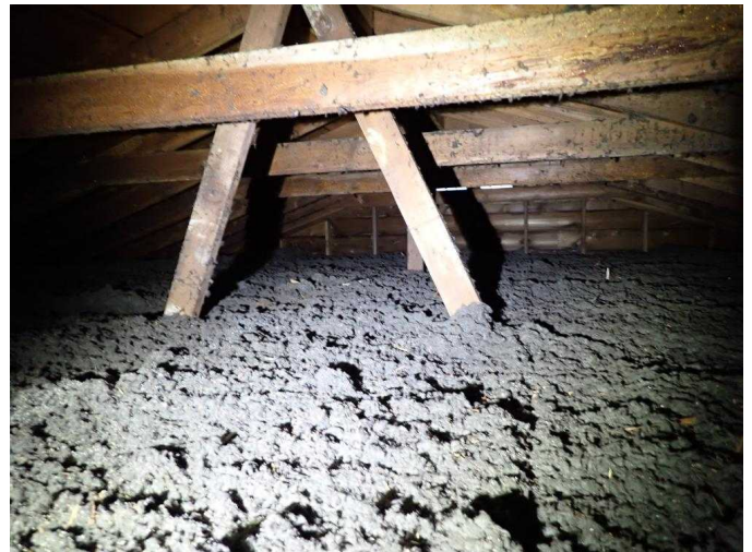
#40 No lower intake ventilation present, reduced air flow in attic space, normal for age of house.
