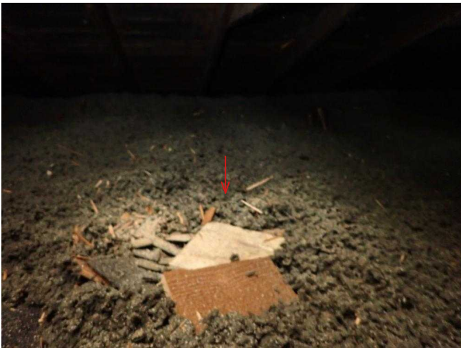
#39 Light amount of roof debris noted in attic.
