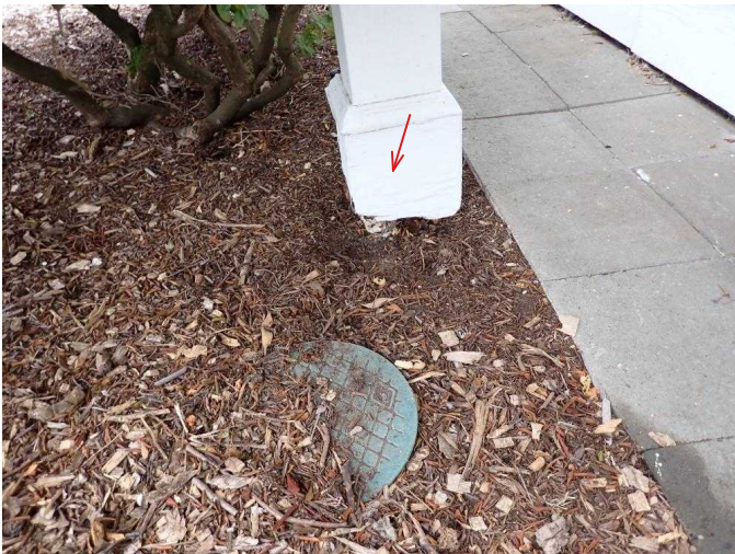
#3 Rot occurring in lower ends of E and W front porch roof support pillars.
