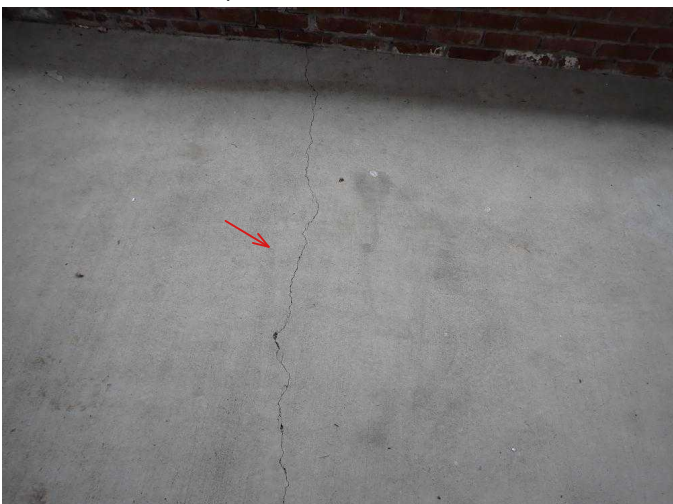
#11 Cosmetic cracks present in patio surface.
