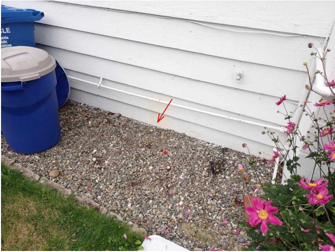
#7 Soil in contact with siding along E side of house, higher potential for rot to occur, soil needs to be removed.
