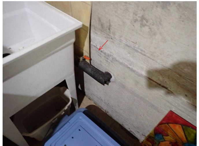
#52 Main water shutoff located in laundry room on N side of laundry sink.
