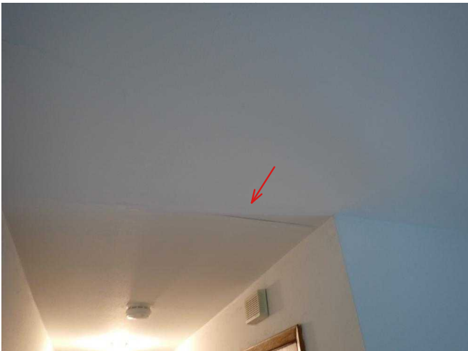
#27 Minor age crack in upper hall ceiling junction with stairwell.
