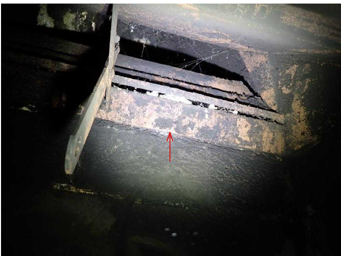
#29 Minor creosote build up in living room smoke chamber, needs to be cleaned before use.
