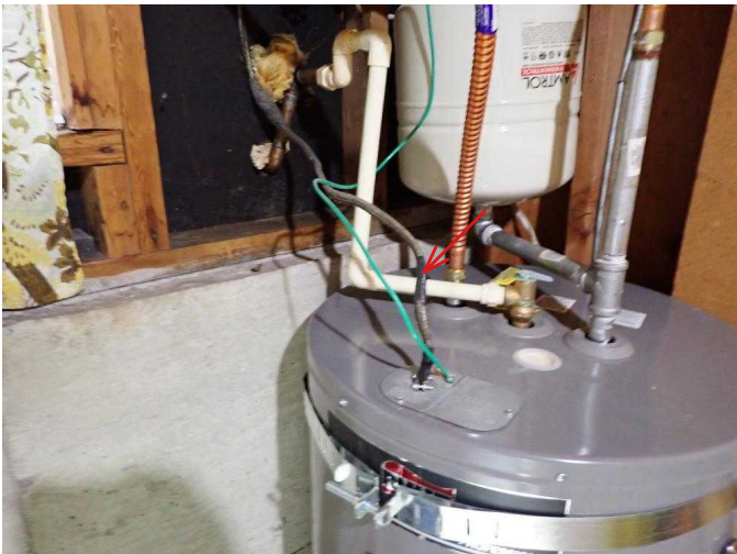
#51 Exposed wiring to water heater needs to be in conduit.
