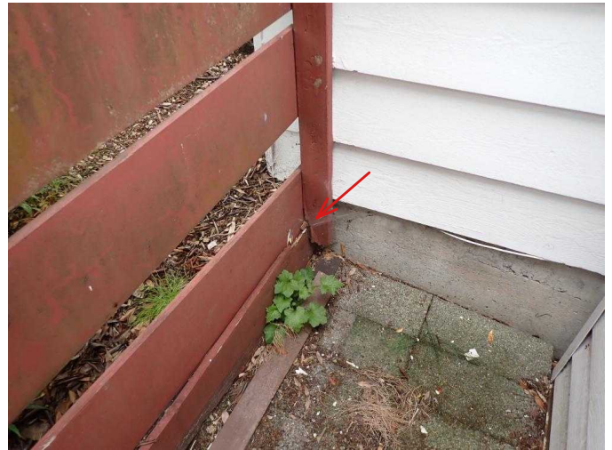
#20 Rot in sections of fence system.
