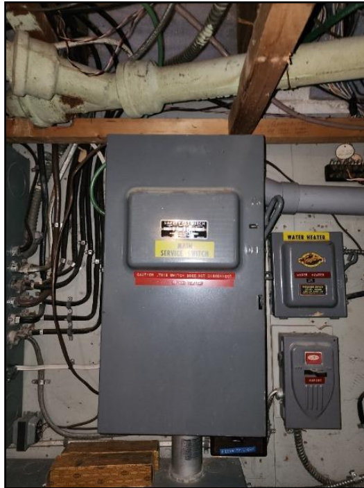
5. Main electrical disconnect
