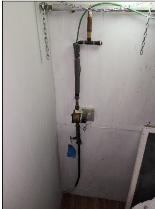
40. Main water shut off
