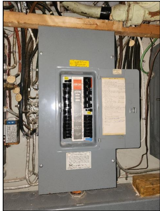
7. Breakers - utility room
