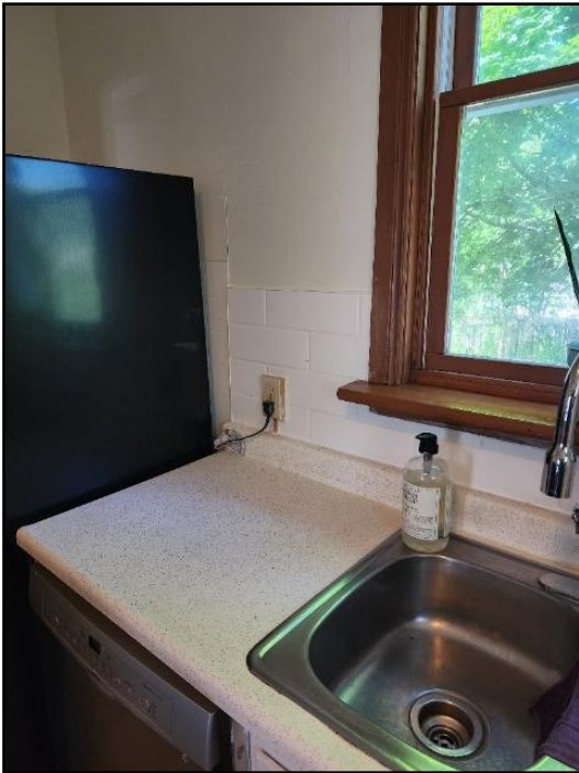
26. No GFCI/GFI (Ground Fault Circuit...
