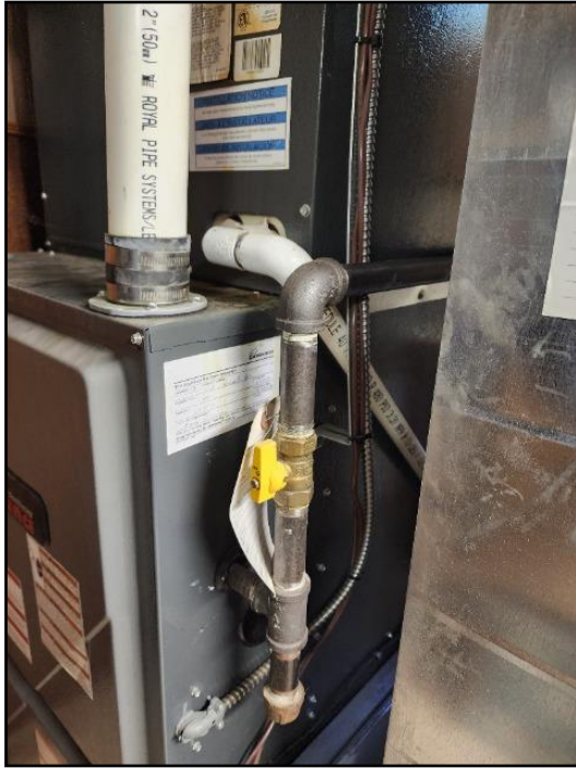
30. Main fuel shut off
