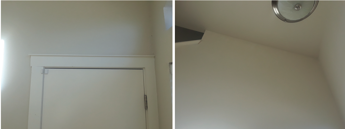
Pictures I1 - I2: Minor out-of-square door at the front entry. Interior doors opened, closed and latched within reasonable expectations. Minor sheetrock cracking various locations.
