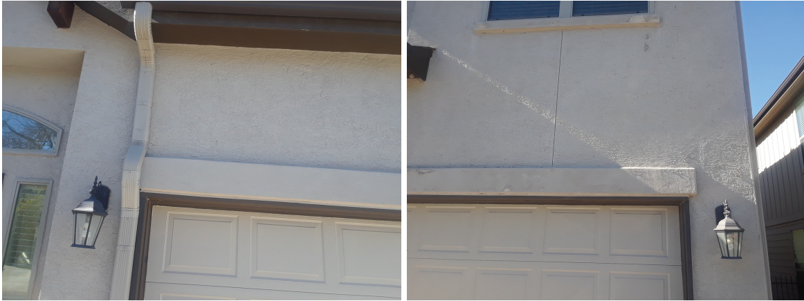
Pictures E5 - E6: Minor stucco and trim separations in various locations.
