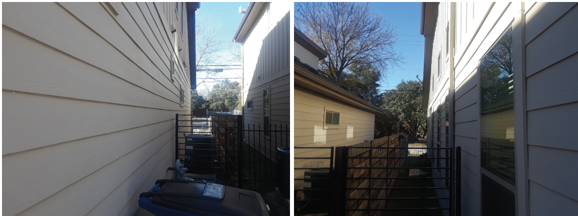
Pictures E1 - E2: Sight down the siding lines along the left and right sides showed siding line deflections.
