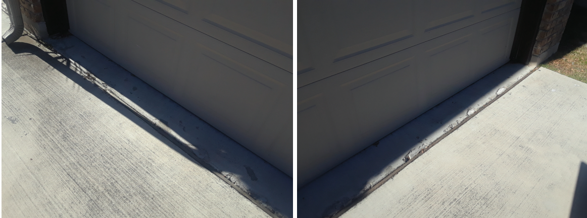
Pictures E3 - E4: No vertical driveway/garage displacement.
