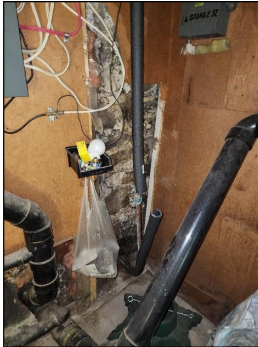
31. Main water shut off
