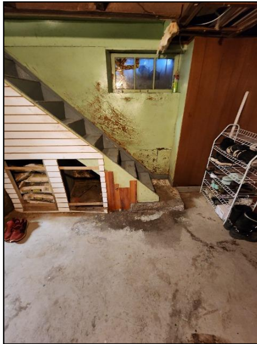
38. Dampness on floor or walls
