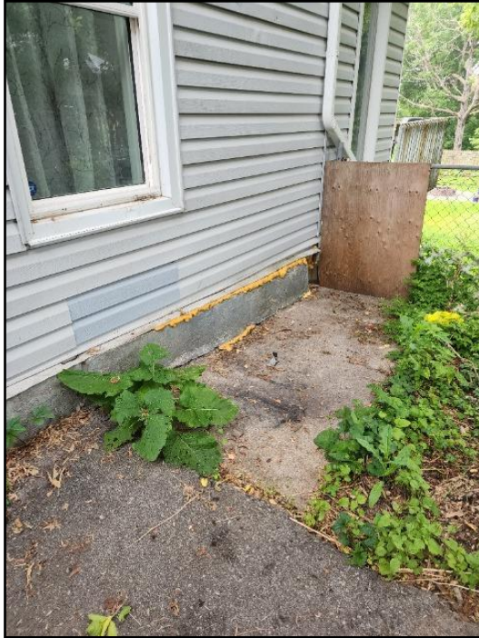
9. Typical minor cracks
