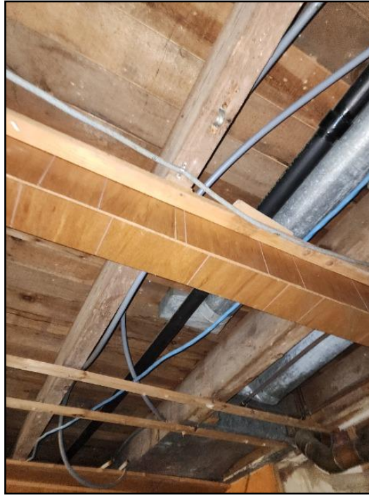
35. Polybutylene Polybutylene has been replaced
