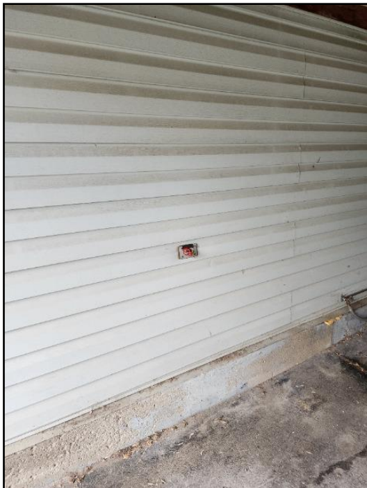
16. No GFCI/GFI (Ground Fault Circuit...
