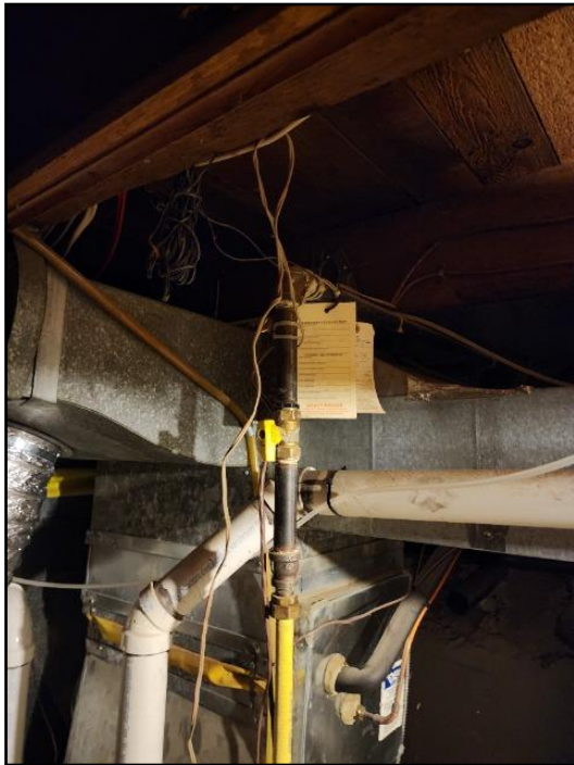
22. Main fuel shut off
