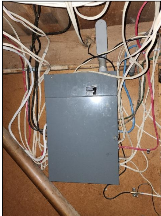
12. Main electrical disconnect
