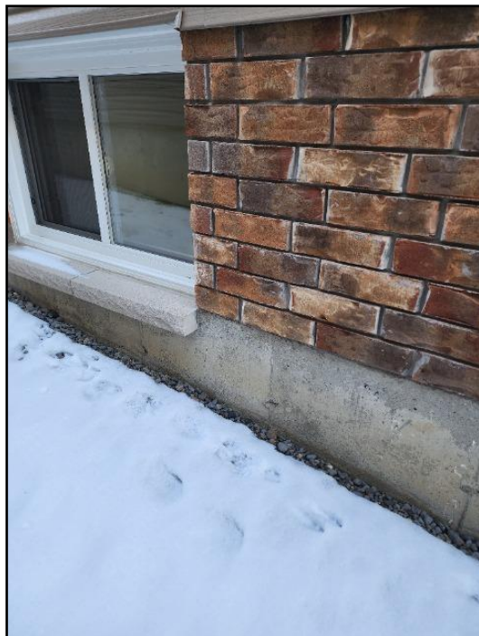
2. Typical minor cracks
