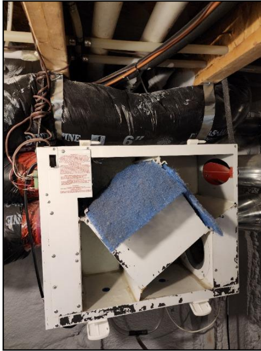
16. Clean filters - regular maintenance
