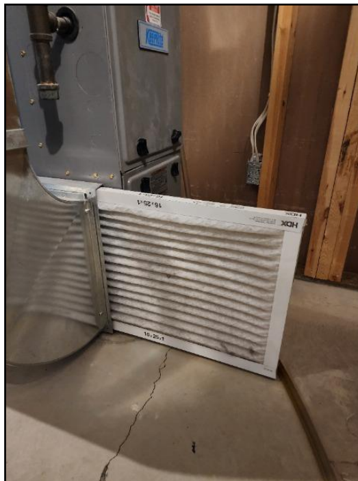
13. Replace - regular maintenance
