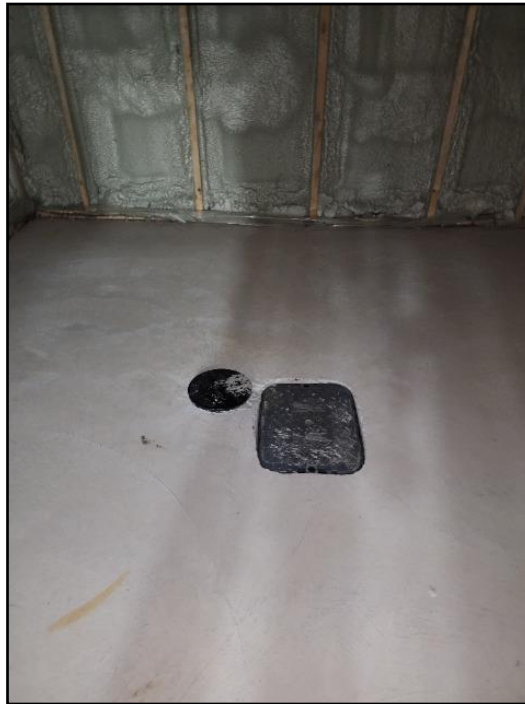
27. Present. These valves help prevent sewer...
