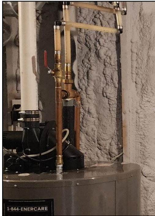
23. Tempering/mixing valve installed
