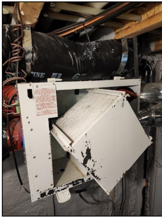
15. Clean core - regular maintenance
