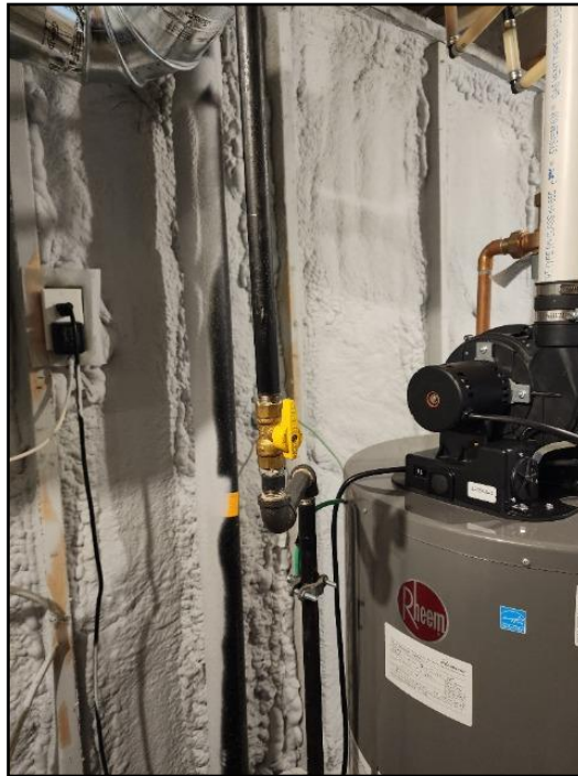
26. Main fuel shut off
