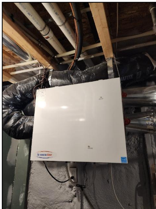
12. Heat recovery ventilator (HRV)
