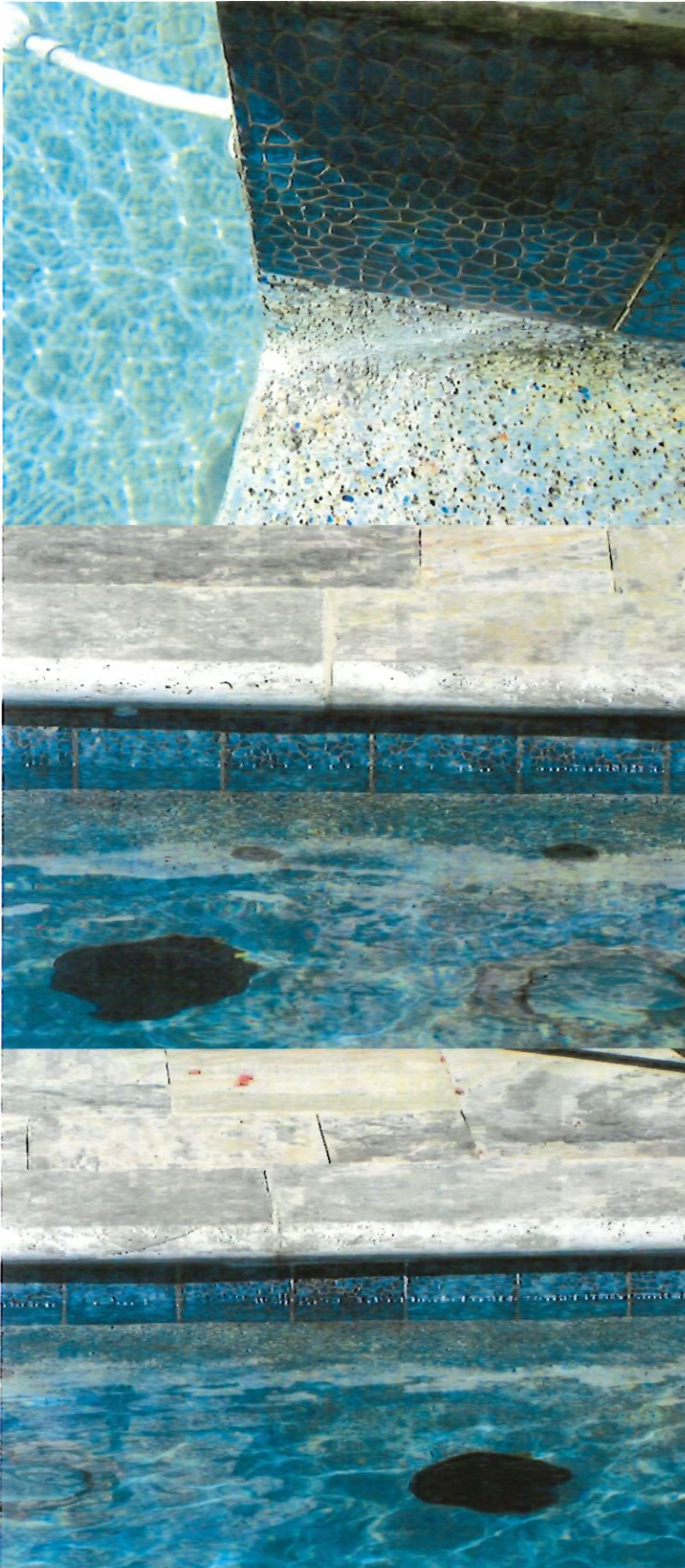
40. Crack in pool shell at southeast corner of tanning area.
