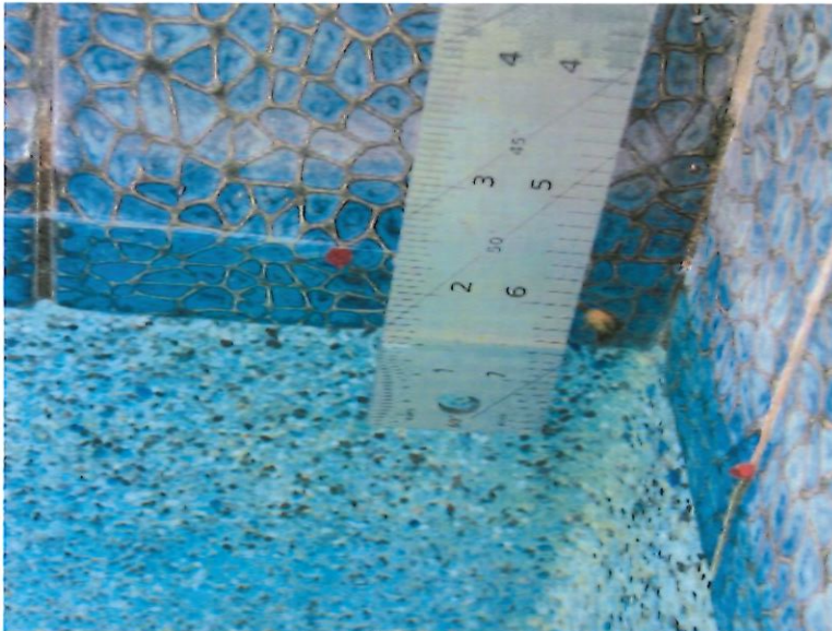
13. Water level at pool at east side of spa at northeast corner measures 6-1/2" below top of coping.
