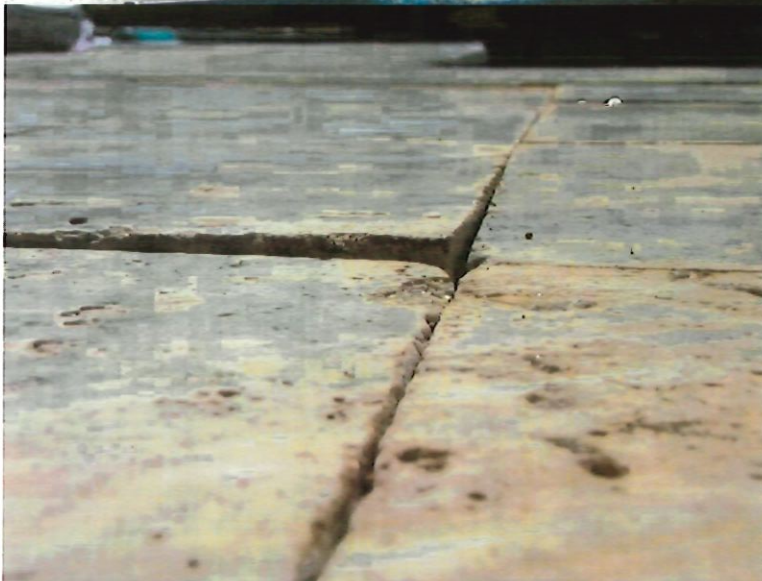
29. Diselevation at paver along west side of tanning area.
