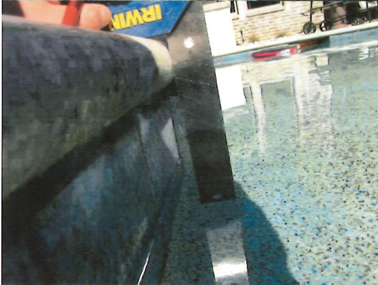
8. Water level at east side of fireplace measures 5-3/4" below top of coping.
