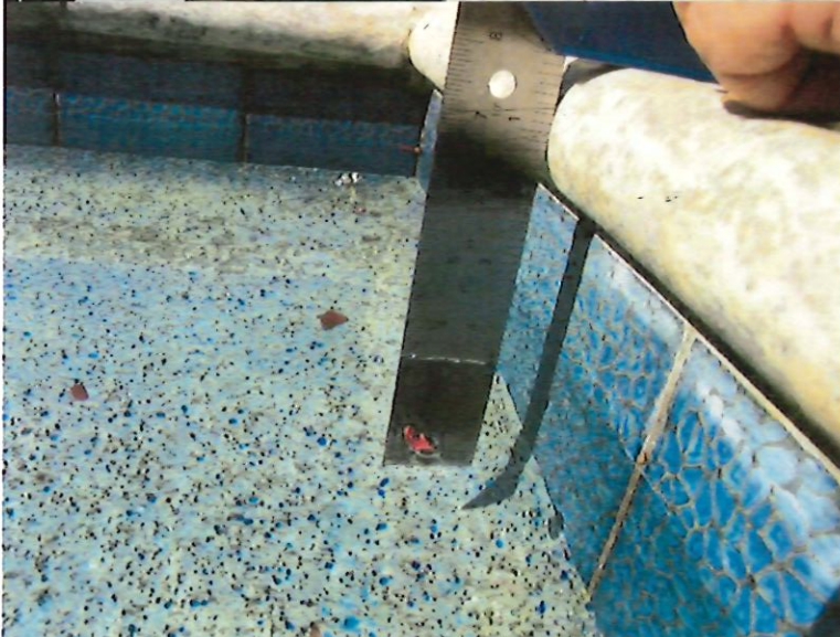
6. Water level at southwest corner of pool measures 4.5" below top of coping.
