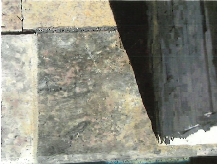
28. Cracked coping tile at same location from prior photograph.
