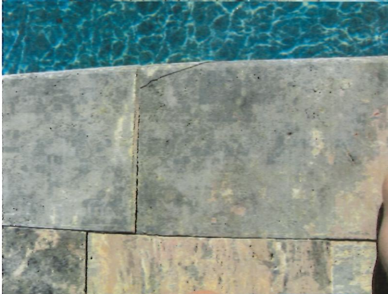
38. Cracked coping ledge at southwest corner of pool.
