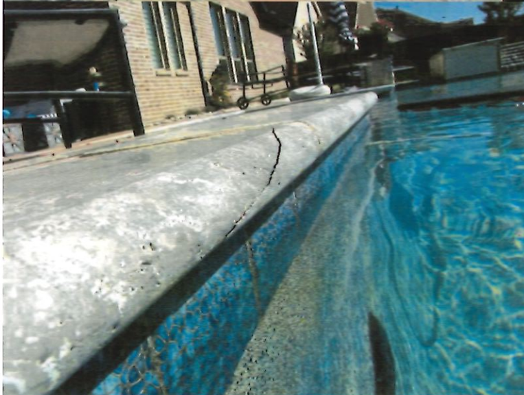
39. Cracked coping ledge at southwest corner of pool.
