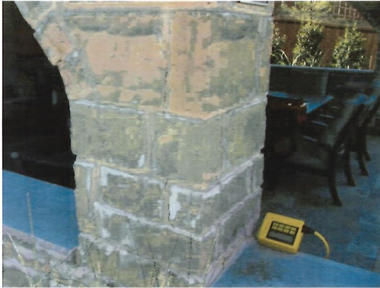
52. Mortar separation at northwest column of gazebo.
