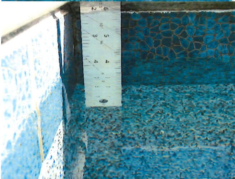
17. Water level at northwest corner of spa measures 4-5/8" below top of coping.
