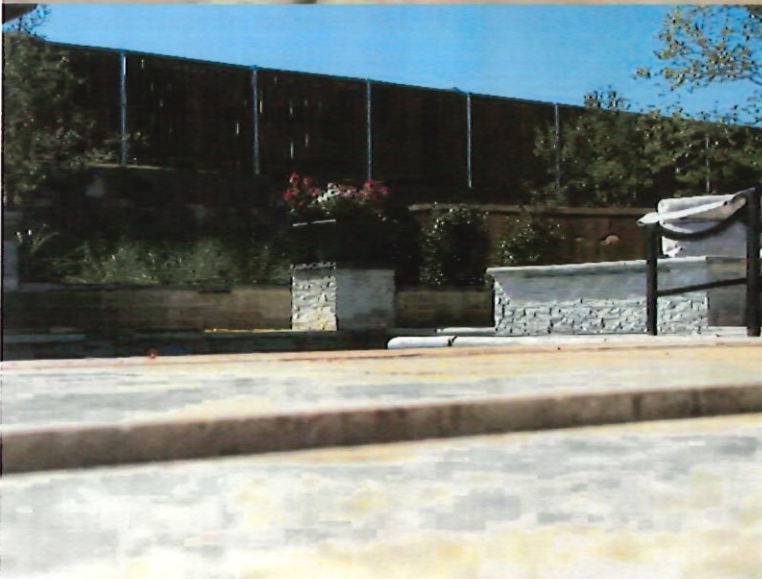
30. Diselevation at paver along west side of tanning area.
