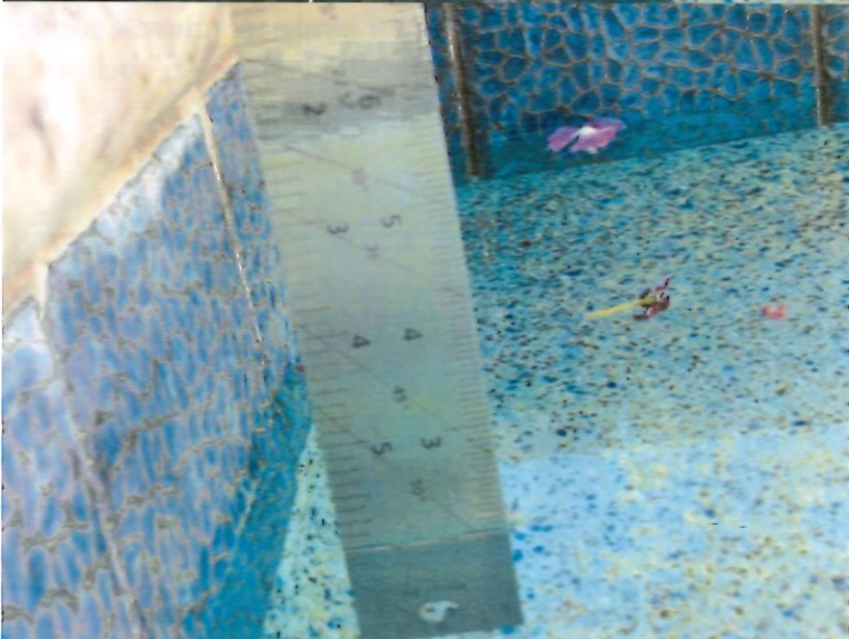
9. Water level at southeast corner measures 6" below top of coping.
