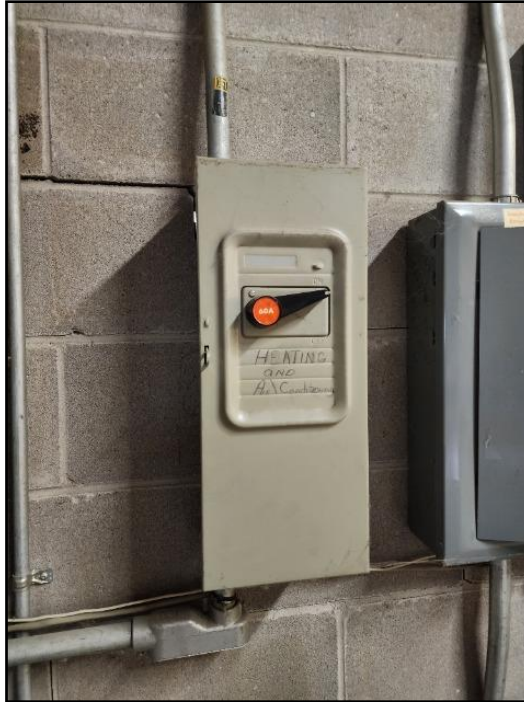
13. Main electrical disconnect
