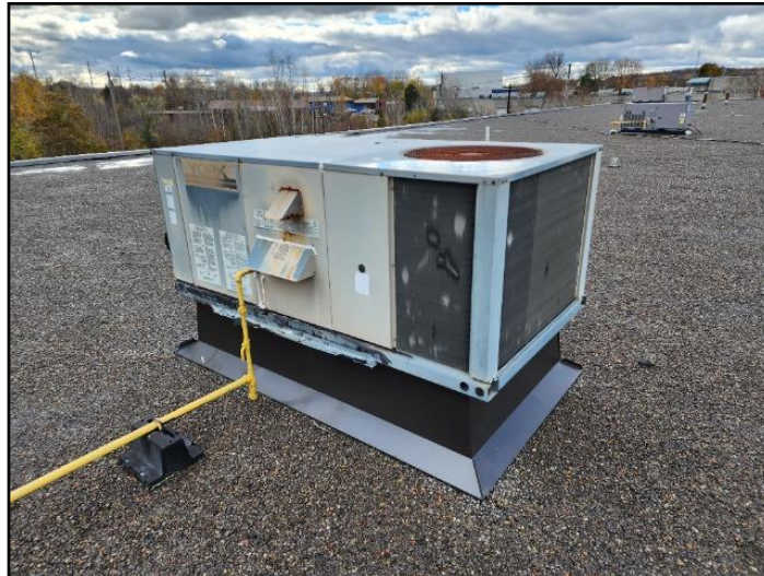
12. Forced air furnace with cooling unit
