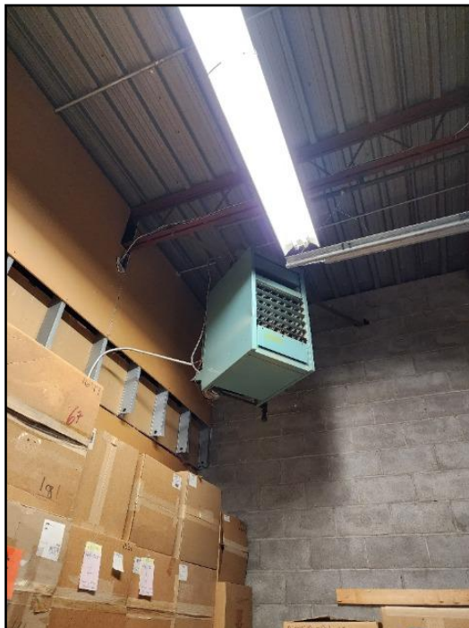
14. Gas space heater
