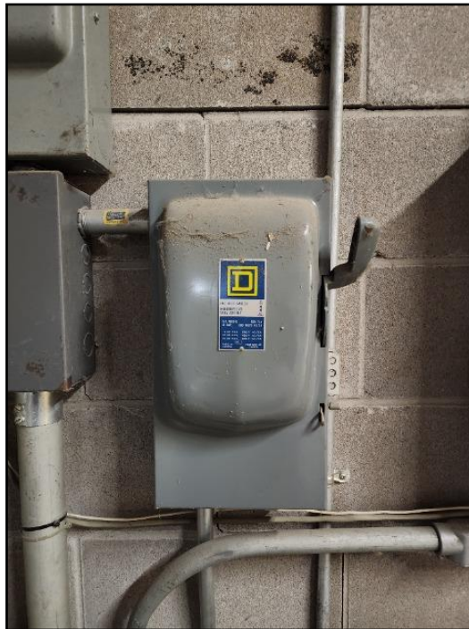
8. Main electrical disconnect
