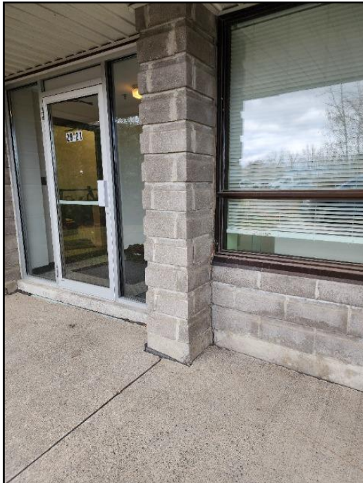
5. Columns/piers settling or shifting
