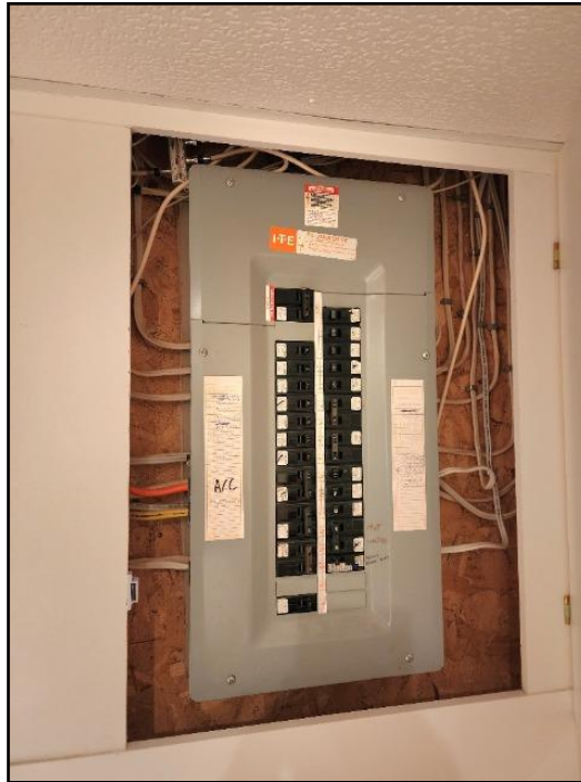
5. Main electrical disconnect
