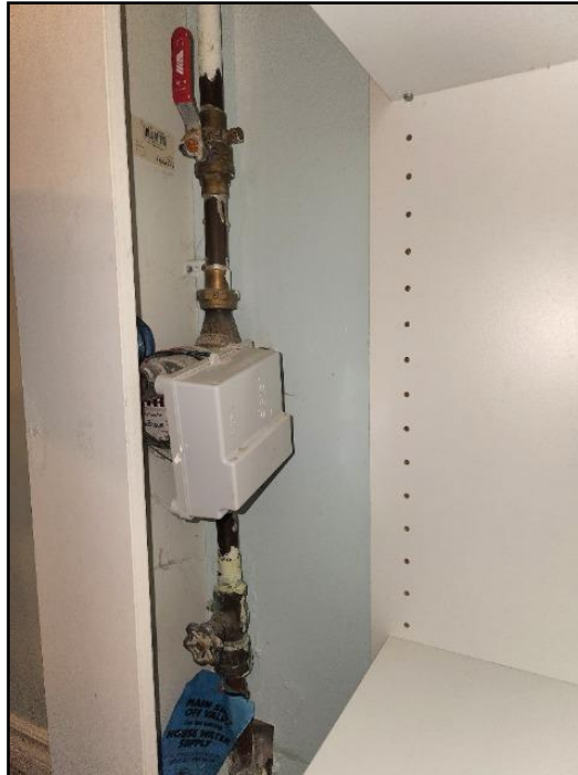
20. Main water shut off
