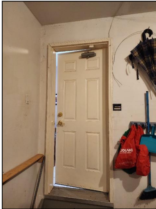
28. Self closer missing, damaged or disconnected
