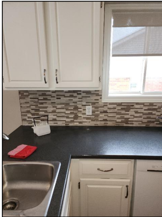
7. No GFCI/GFI (Ground Fault Circuit...
