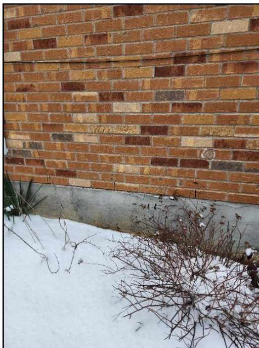
1. Typical minor cracks
