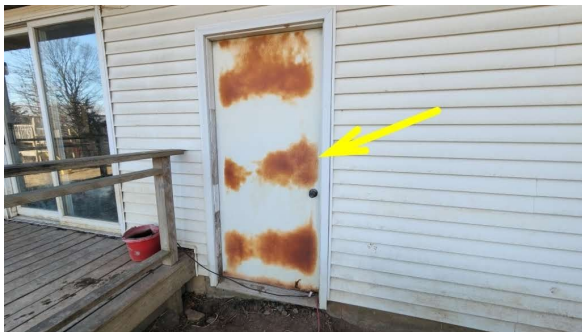
North garage walk door has rusted, deteriorated.
