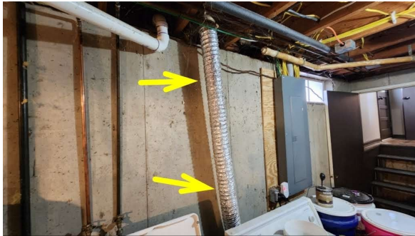
Recommend replacing flexible dryer vent with rigid vent rated for gas dryers.
