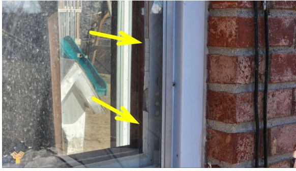
Loose and missing glazing, peeling paint observed throughout wood windows. Examples above.
