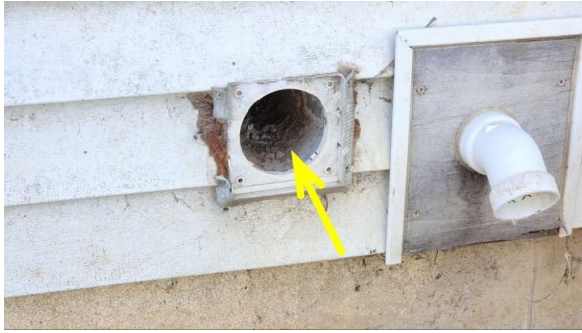
Dryer vent damper was missing. Recommend installing.
