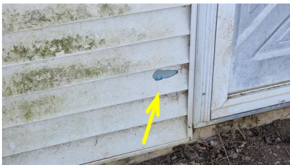
Northeast vinyl siding was damaged along the lower course.
