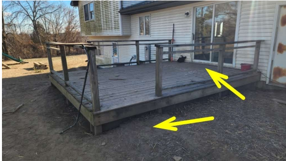
Deck guardrail spindles were spaced greater than 4 inches. West step was steep (rise greater than 7 inches).
