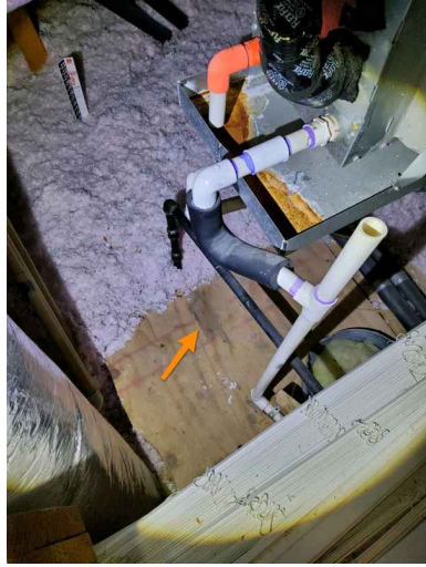
Below The West Unit In The Attic
