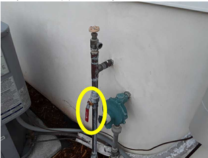
The local water shut-off valve is located at the rear of the home, unit, or building.
