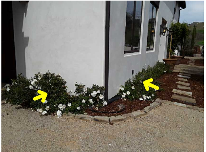
Vines, shrubs or bushes are growing on the house walls and although they are attractive they can introduce pests and rodents and accelerate deterioration. Therefore, you may wish to consider having them removed or cut back to 12 inches (30 cm) away from the home.
