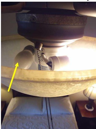
A ceiling light bulb in the bedroom does not respond, and should be serviced.
