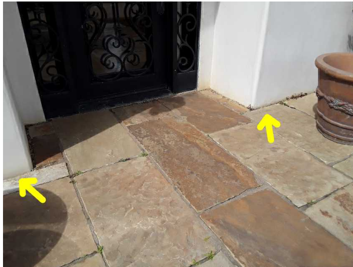
Portions of the weep-screed have been covered. Weep-screed not only allows the house walls to move independently of the foundation and prevents the plate-line cracks that are commonly seen at the base of many stucco walls but allows any moisture that penetrates the stucco to drain. Therefore, the interior and exterior plaster in this area should be monitored to ensure that no moisture damage results.
