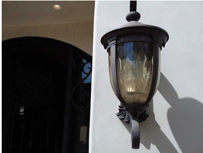
An exterior wall light did not respond and should be serviced.
