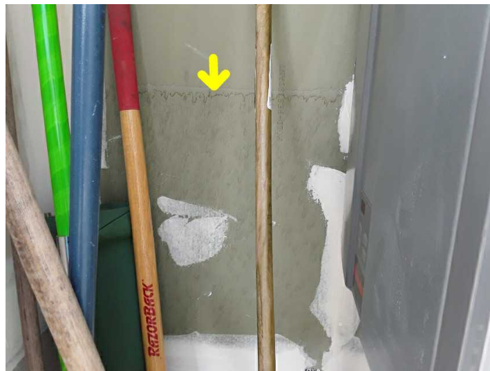
There is a moisture stain on the wall or ceiling that should be explained or explored further.
