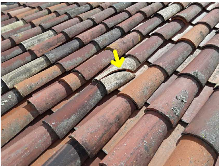
There are cracked or broken tiles that should be serviced by a licensed roofing contractor.
