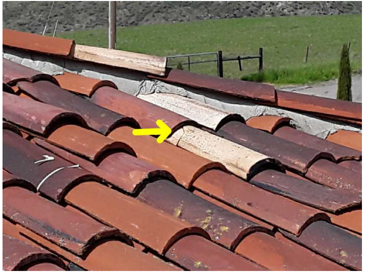
There are cracked or broken tiles that should be serviced by a licensed roofing contractor.
