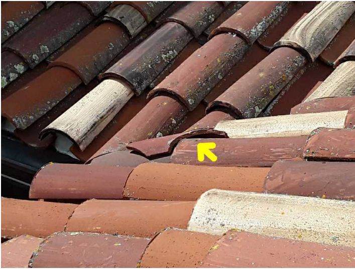
There are cracked or broken tiles that should be serviced by a licensed roofing contractor.
