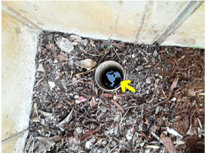
There is standing water or debris visible within the area drains, which could be indicative of at least a partial blockage. The tendrils of roots may have invaded the drains, but silt also tends to become trapped within the drain pipes and hardens during the summer months to the consistency of wet concrete and creates an impediment that commonly leads to a full blockage. Therefore, we recommend that the lines be flushed through to the street or to their termination point.
