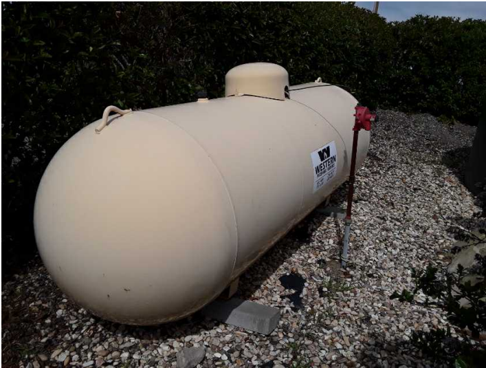
The gas main shut-off is located at the propane tank.
