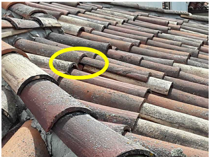
There are cracked or broken tiles that should be serviced by a licensed roofing contractor.
