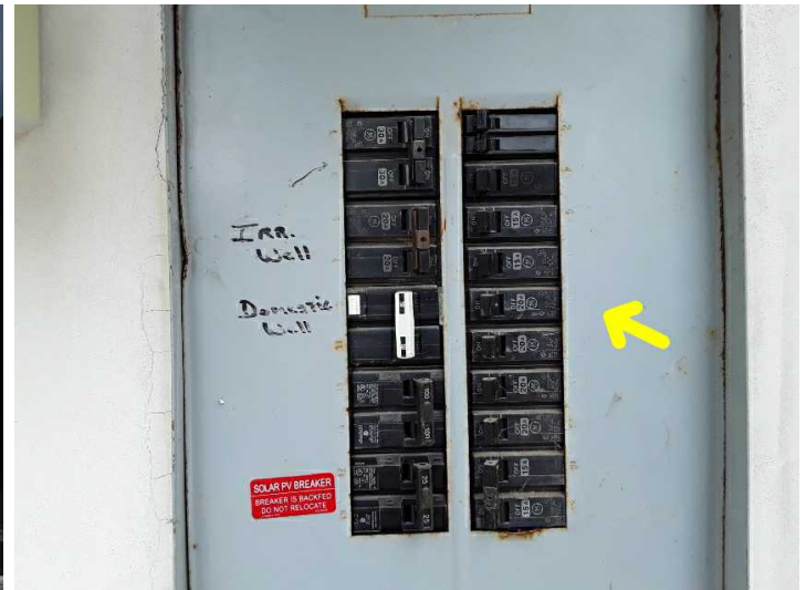
Various circuits within the sub-panel are not labeled, and this condition should be serviced by a qualified electrical contractor so that the appropriate load calculations and breaker sizes can be determined.
