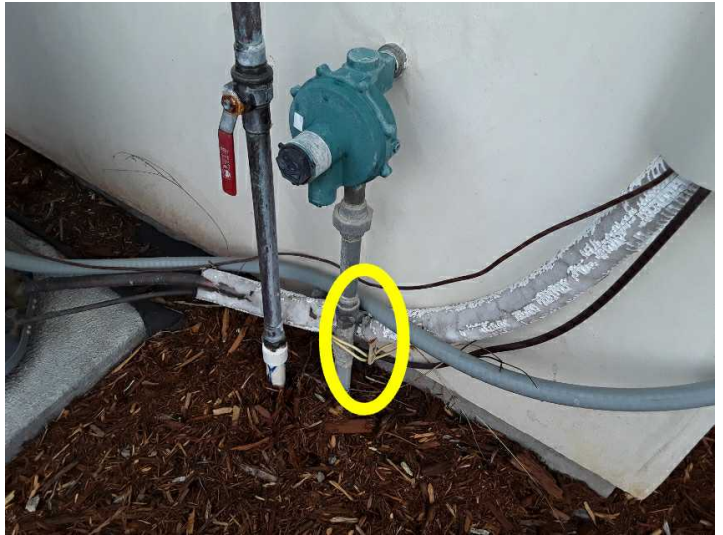
The local gas shut-off is located on the rear of the home, unit or building.
