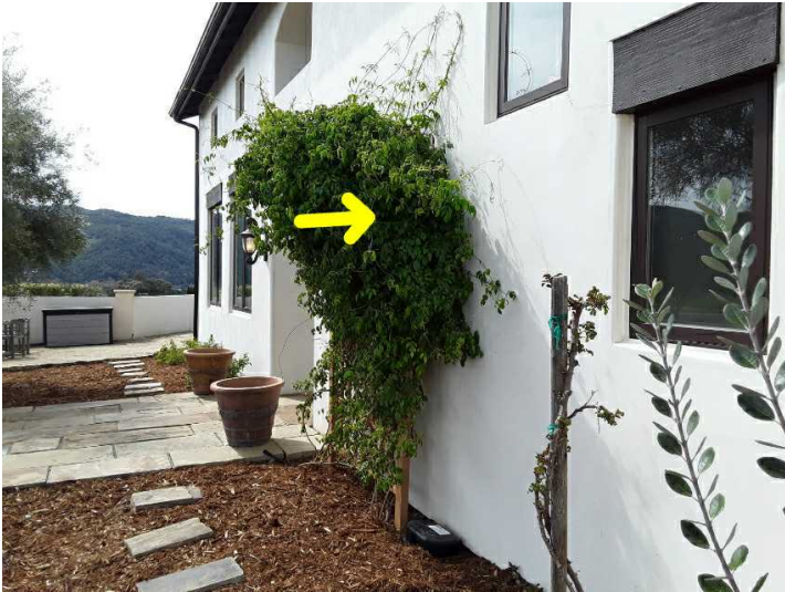
Vines, shrubs or bushes are growing on the house walls and although they are attractive they can introduce pests and rodents and accelerate deterioration. Therefore, you may wish to consider having them removed or cut back to 12 inches (30 cm) away from the home.
