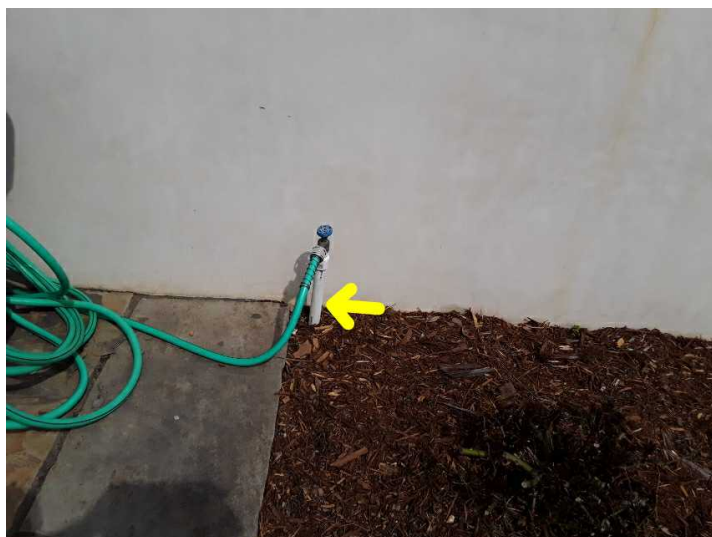
A PVC hose bib pipe should be braced with a metal stake to reduce the possibility of leaks.
