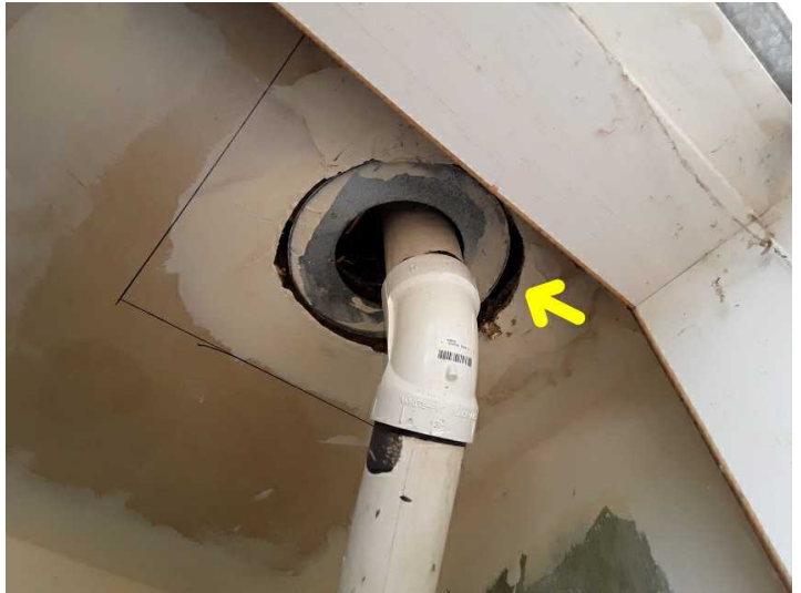
A transition spacer is improperly sized where the vent pipe enters the attic or wall cavity, which should be serviced.
