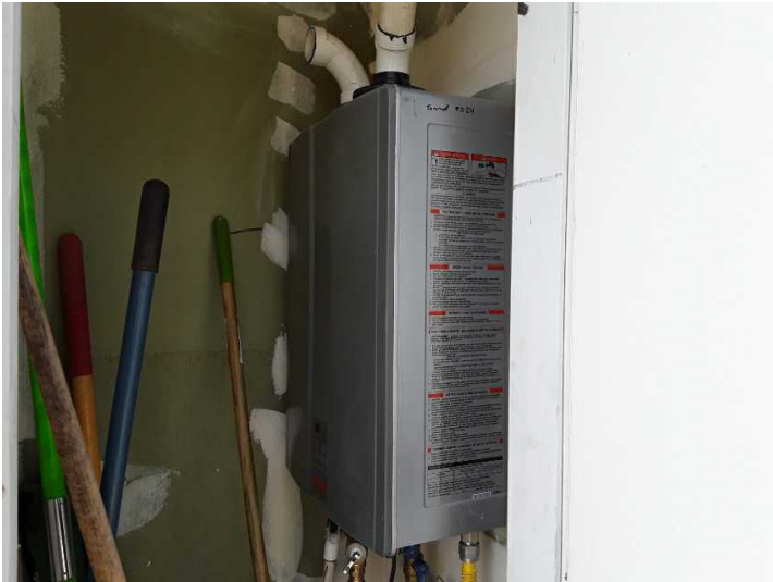
The residence is served by a tankless water heater located in an exterior closet.
