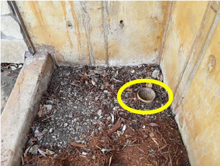
There are missing or broken area drain covers. This could have allowed leaves and other debris to enter the drain lines and contribute to blockages. Therefore, it would be prudent to have the lines flushed through to the street or to their termination point before the broken covers are replaced.
