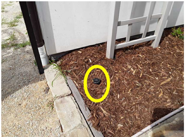
There are area drains in planter beds or yards that will be subject to contamination by dirt and debris, and these drains should be periodically monitored and cleaned.
