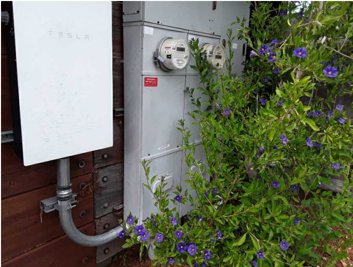
The residence is served by a 200 amp main electrical panel, located at the rear of the home or unit.
