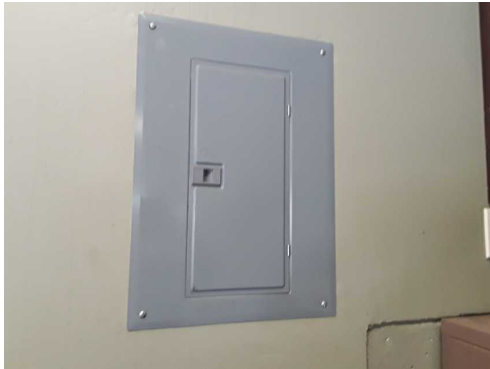
The sub panel is located within the garage.
