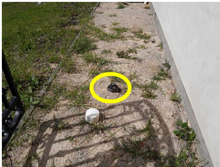
A clean-out is located at the left side.
