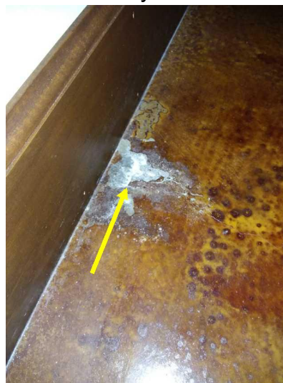
The floor is worn or cosmetically damaged, which you should view for yourself.
