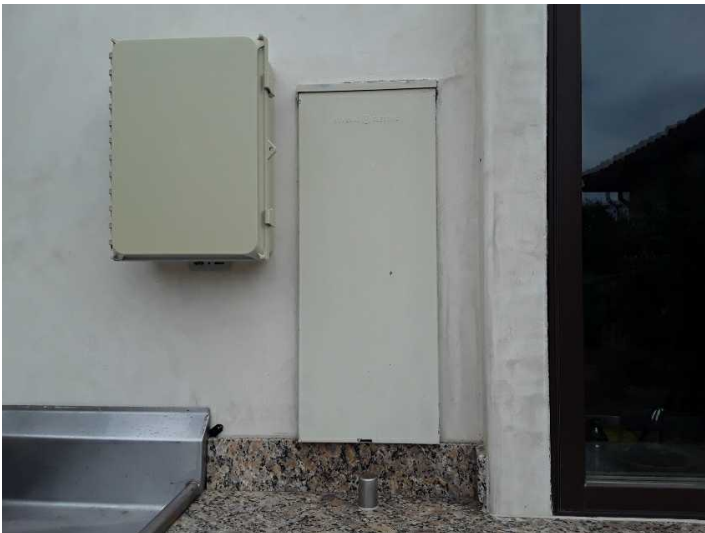
The sub panel is located at the rear exterior of the home.
