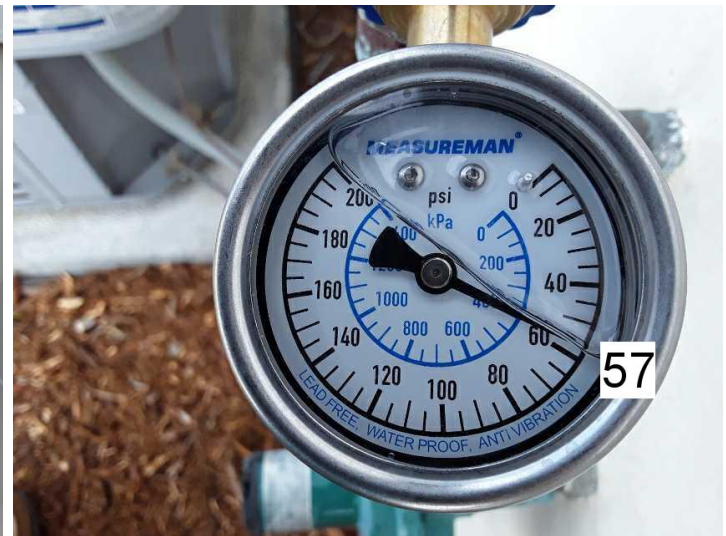
The water pressure entering the residence is under 80 PSI and a regulator is not required on the plumbing system.
