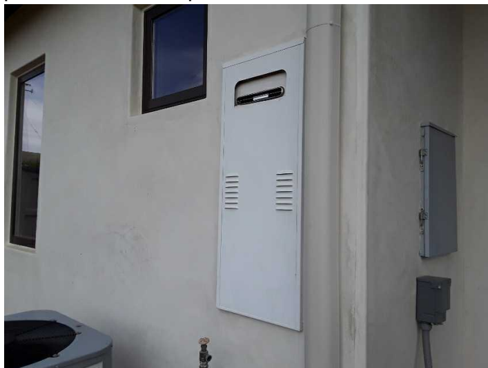
The residence is served by a tankless water heater located in an exterior closet at the rear.
