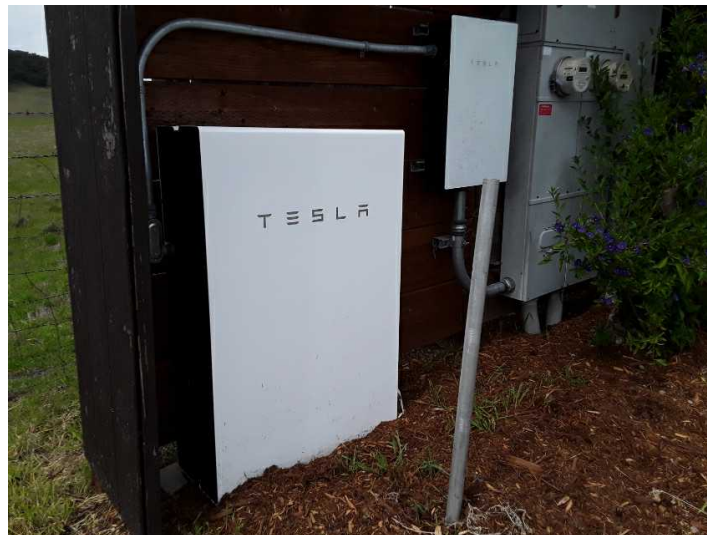
A battery backup or power bank system has been installed, which we do not have the expertise to evaluate. We recommend the sellers provide information regarding its installation, operation, and maintenance history. You may also wish to have it evaluated by a qualified specialist.
