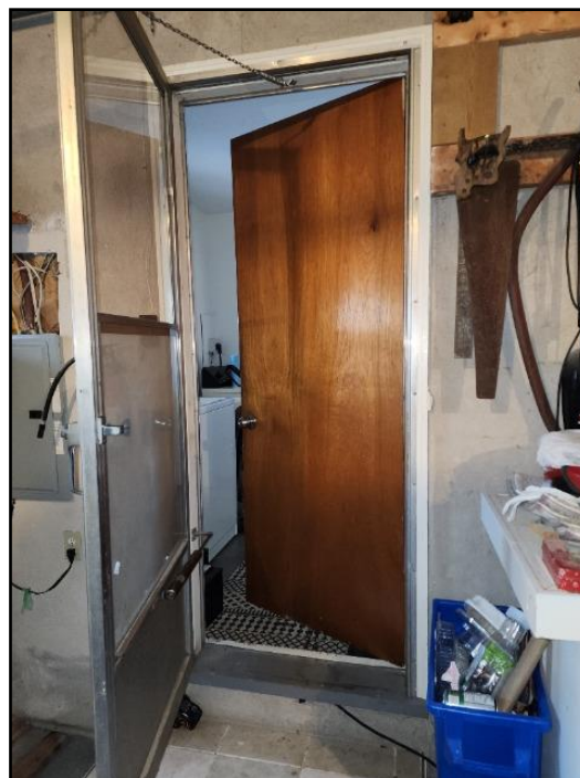
34. Self closer missing, damaged or disconnected
