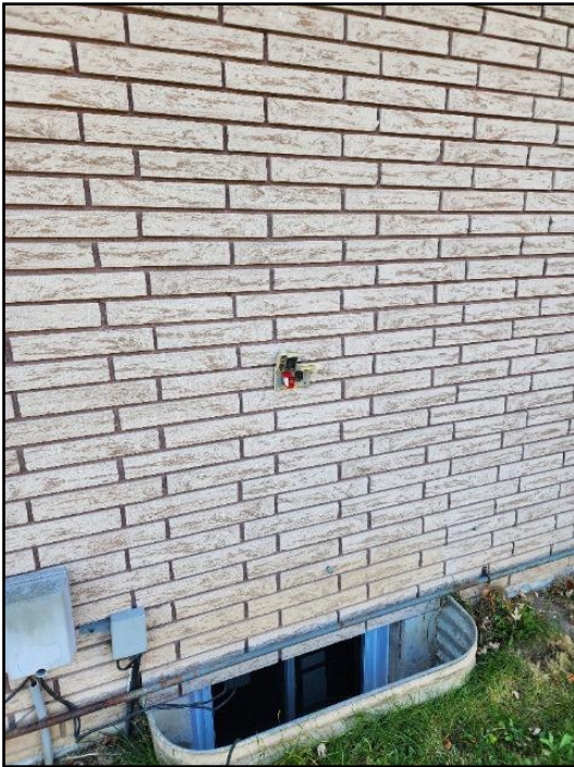
11. No GFCI/GFI (Ground Fault Circuit...
