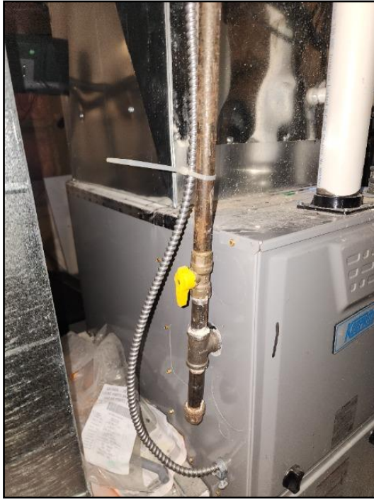
14. Main fuel shut off
