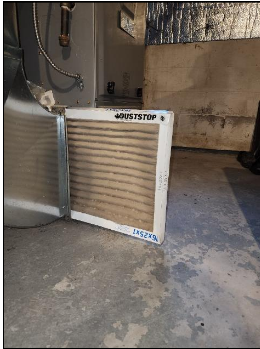
21. Replace - regular maintenance
