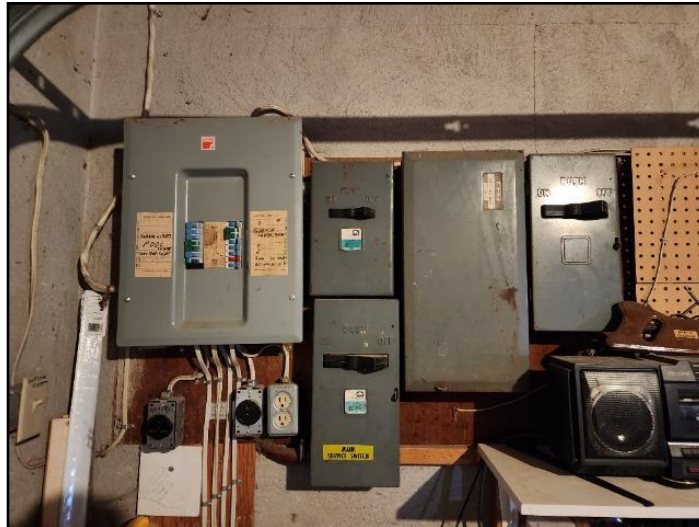
4. Main electrical disconnect
