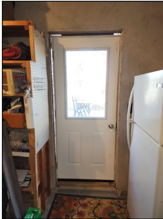
3. Exterior caulk/sealant missing
