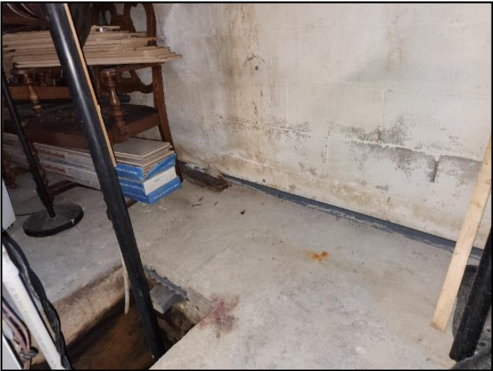
33. Drainage membrane & sump pump
