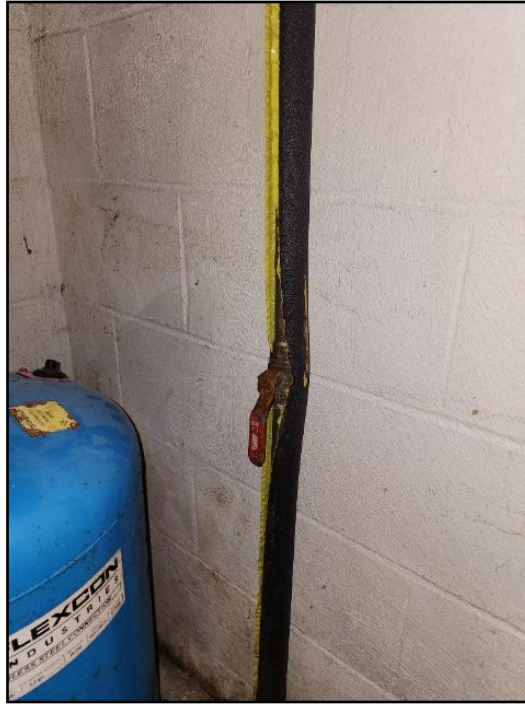
27. Main water shut off
