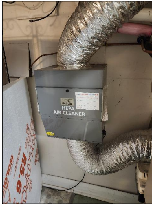
26. HEPA air filtration system
