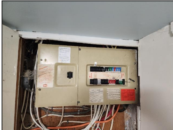
3. Main electrical disconnect
