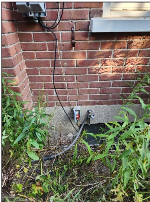
19. No GFCI/GFI (Ground Fault Circuit...)
