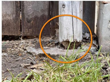
Rotted post/right side, other locations
