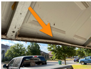
Damaged panels/both doors
