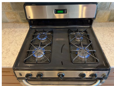
Gas burners Working as Intended
