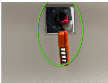
Dryer outlet has power
