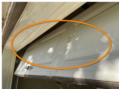
Damaged panels/both doors
