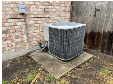
Condensing unit/right side
