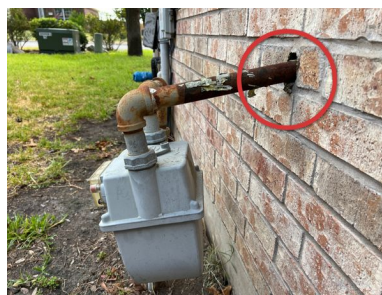
Gas pipe is not bonded
