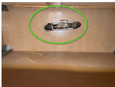
Gas valve/left of the stove
