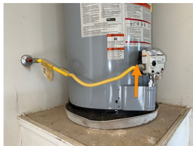
Missing sediment trap
