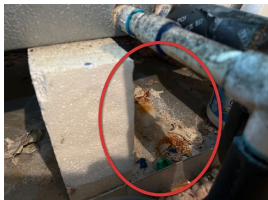
Rust in drain pan
