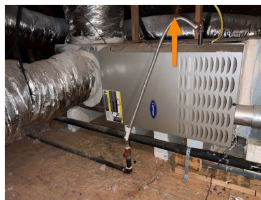
Gas line/missing sediment trap
