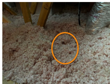
Rodent tunnels in the insulation
