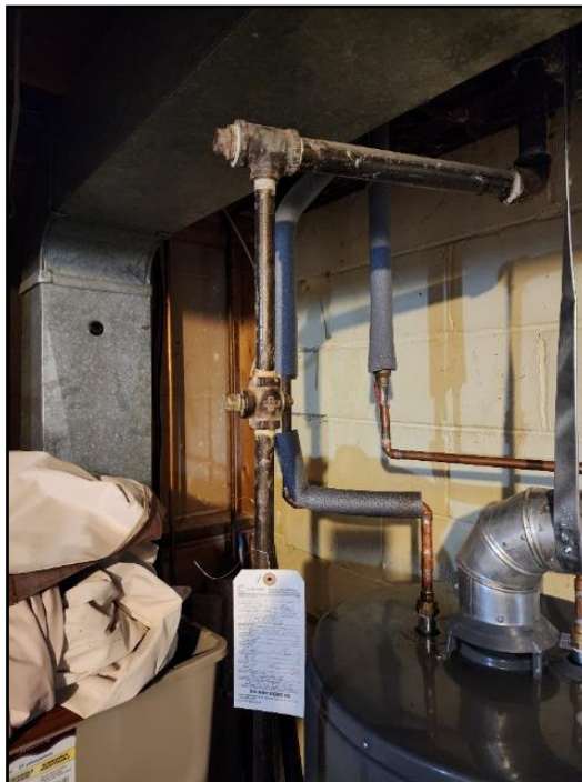
34. Main fuel shut off
