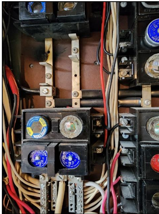
16. Fuses too big
