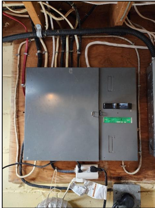
9. Main electrical disconnect
