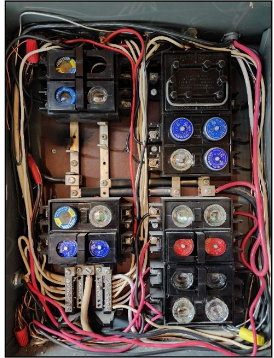
11. Fuses - utility room
