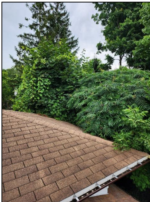
4. Tree branches touching roof
