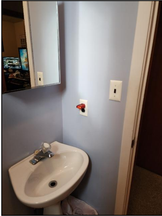
17. No GFCI/GFI (Ground Fault Circuit...
