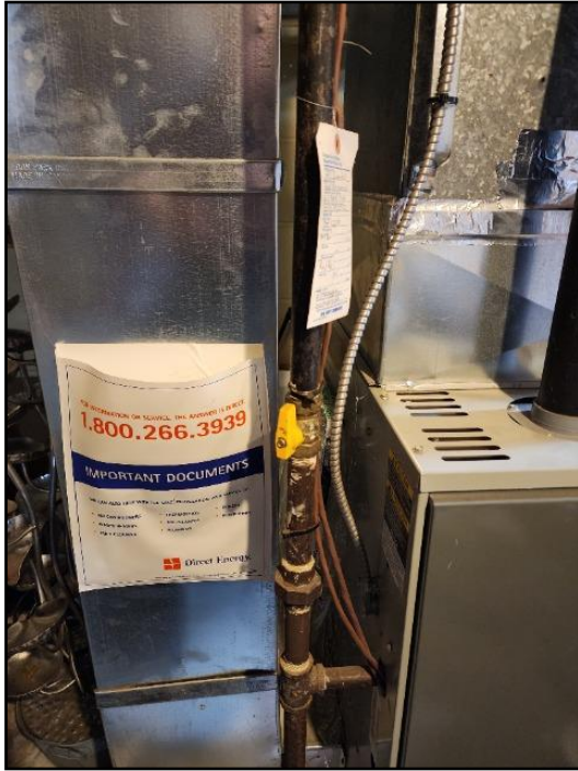
21. Main fuel shut off
