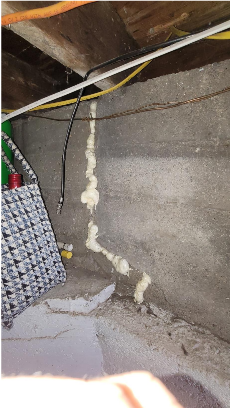
Another shot of the cracking
