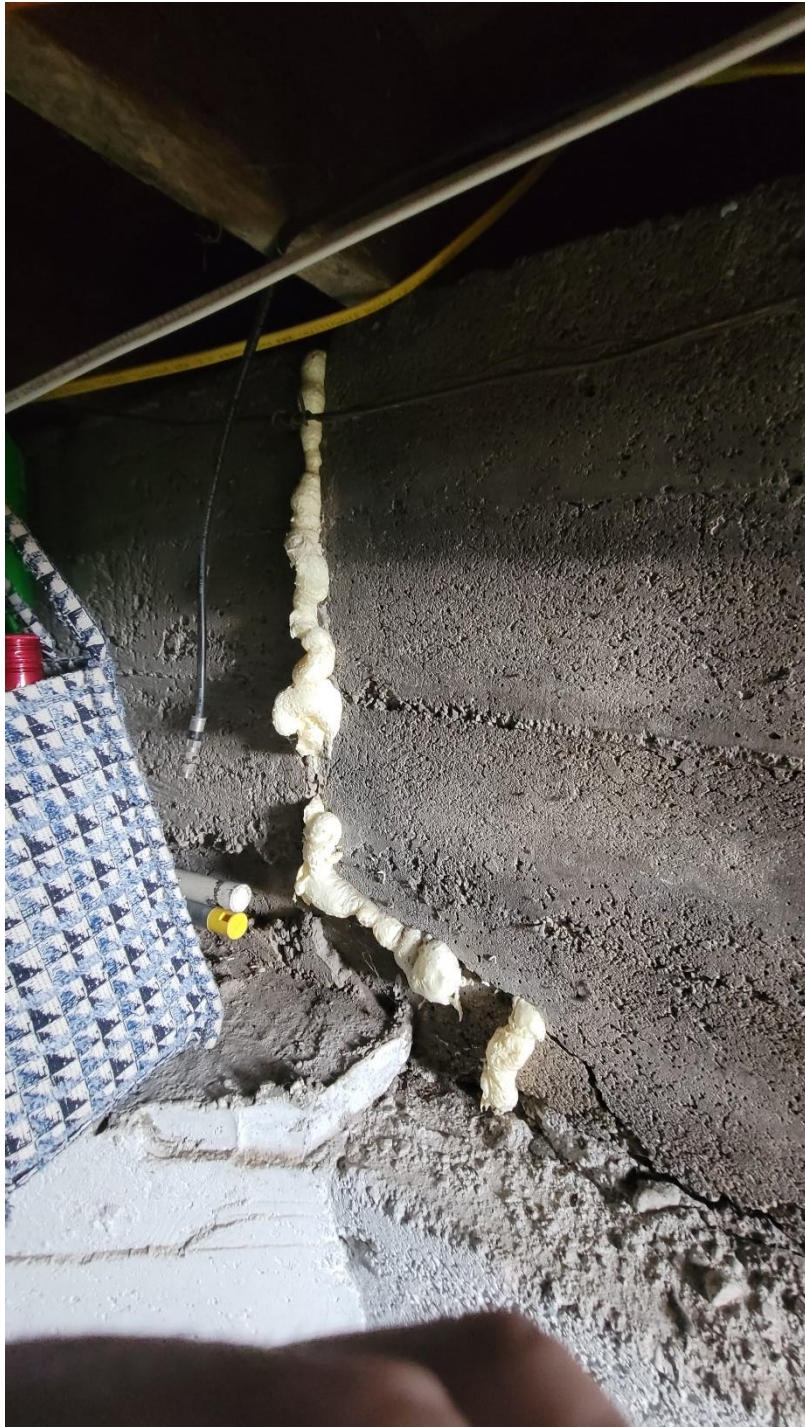
The cracking and expanding foam on the southeast corner
