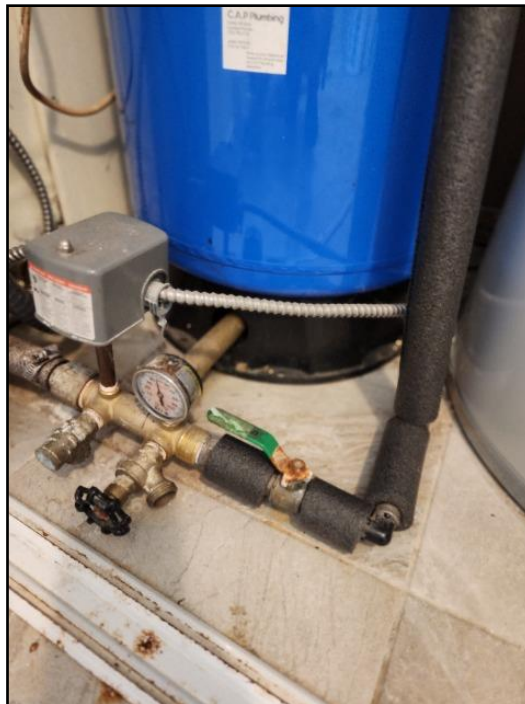
21. Main water shut off
