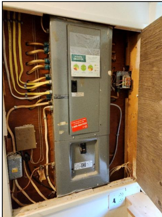
8. Main electrical disconnect
