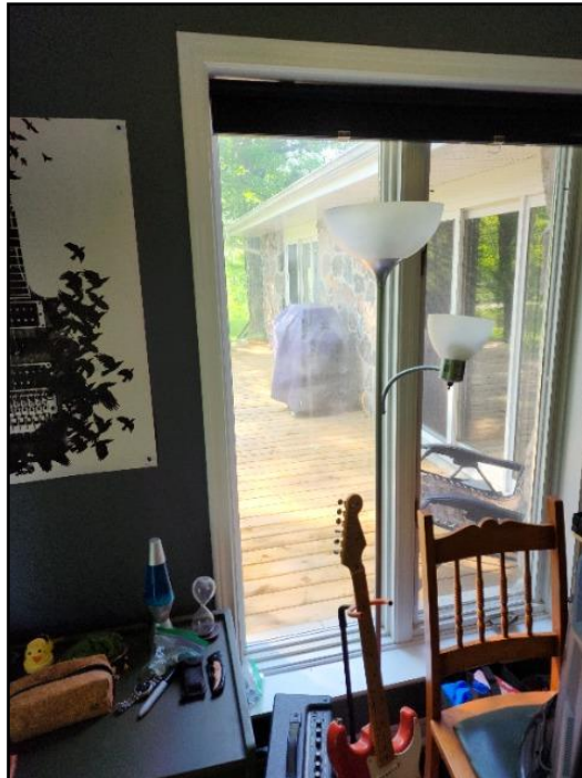
29. Lost seal on double glazing
