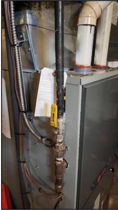
17. Main fuel shut off
