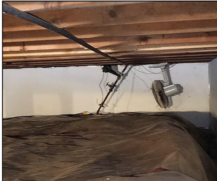
25. Main water shut off
