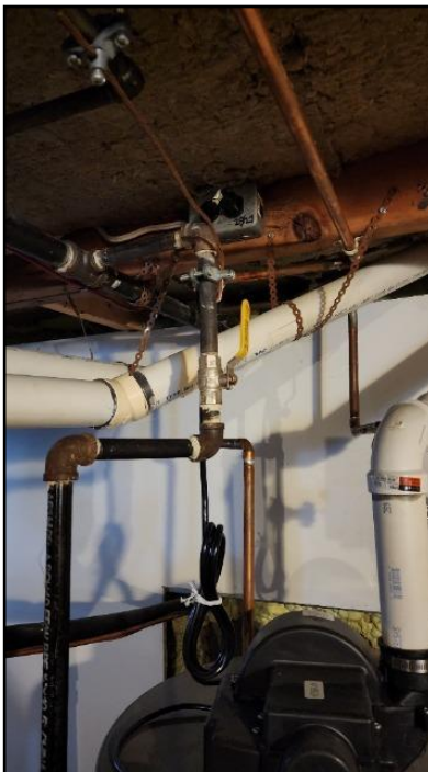
27. Main fuel shut off
