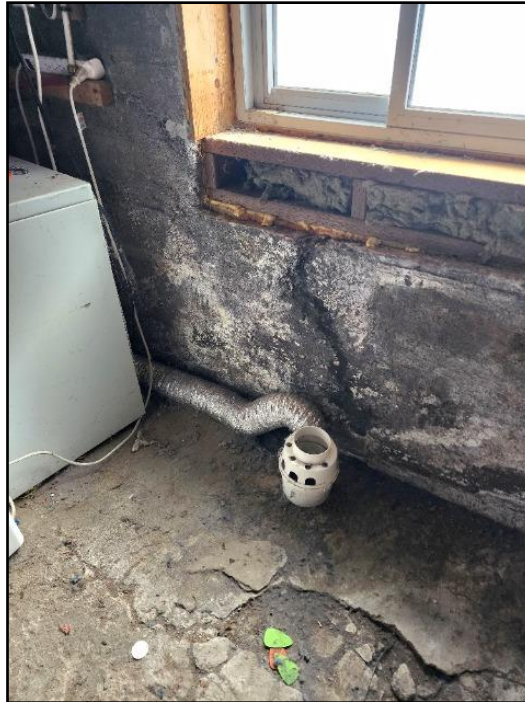
24. Dryer not vented to exterior
