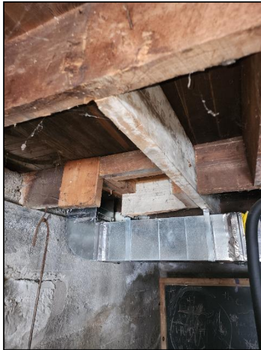
4. Split, cracked or damaged
