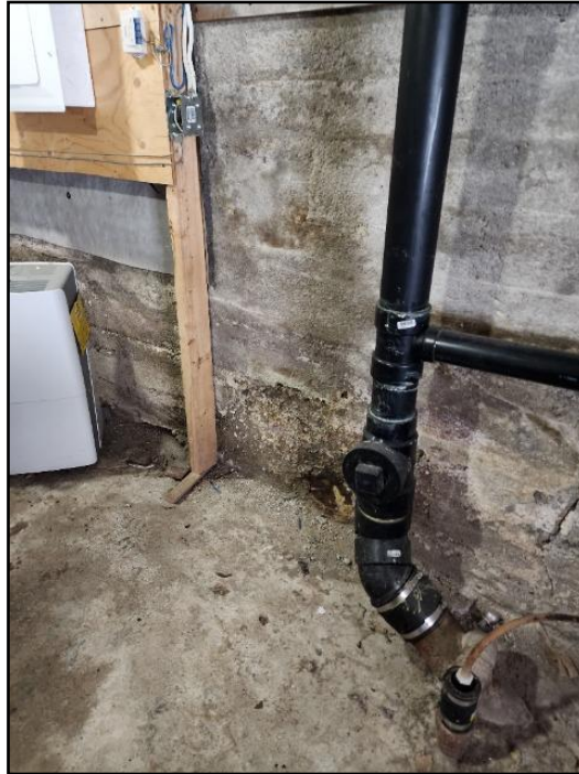
21. Crumbling/spalling masonry, concrete or...
