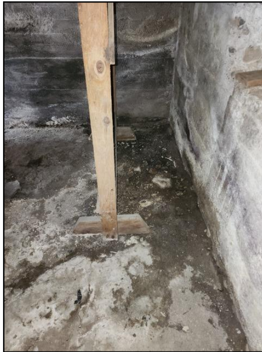
22. Dampness on floor or walls
