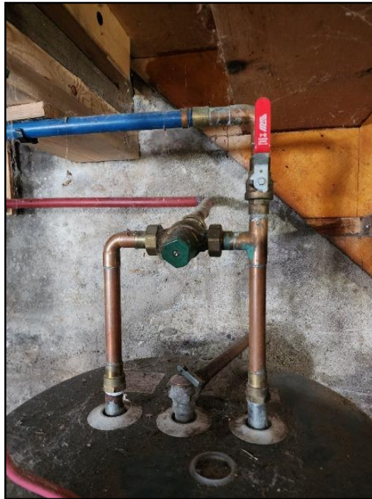
18. Tempering/mixing valve installed
