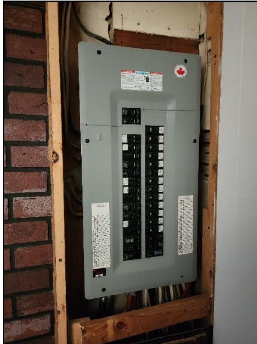
12. Main electrical disconnect
