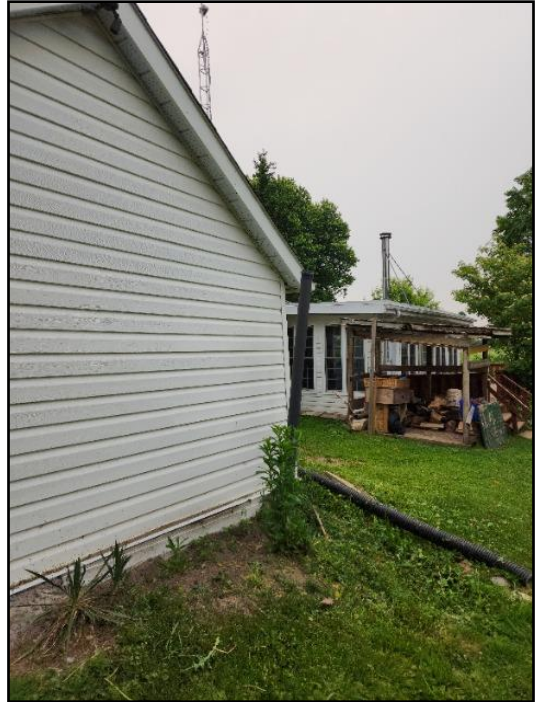
35. Vent termination problems
