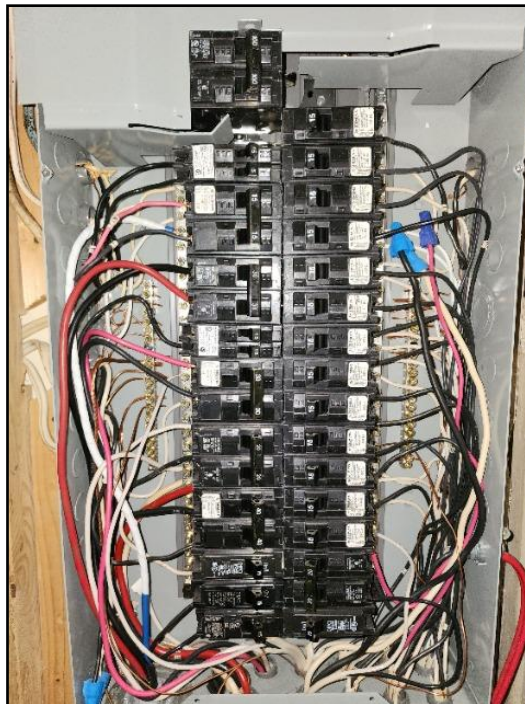
13. Breakers - first floor
