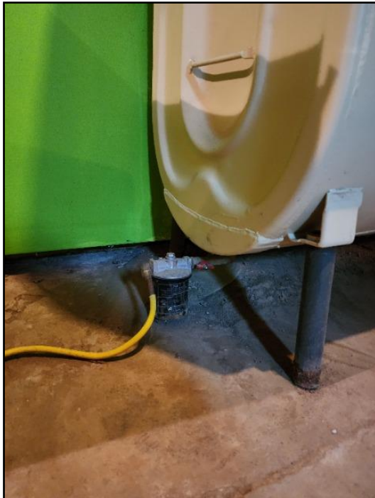
15. Main fuel shut off
