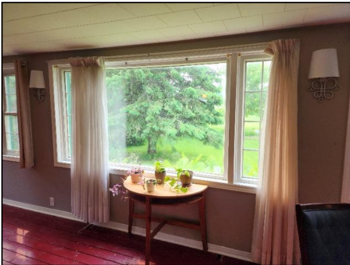
37. Lost seal on double glazing
