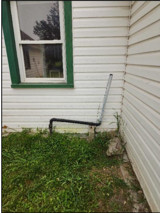
34. Vent termination problems
