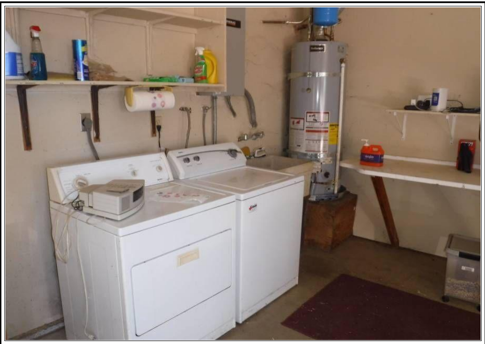
water heater and laundry in garage
