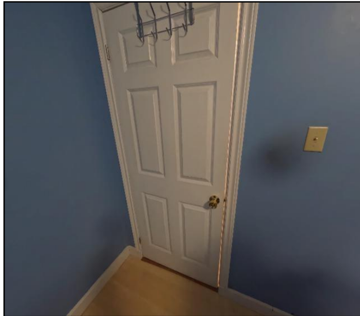
108. Loose or poor fit
