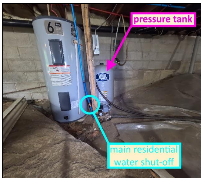
75. Near pressure tank
