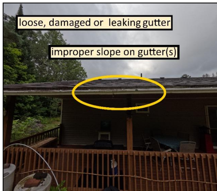
45. Improper slope, ponding
