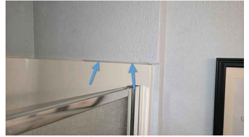
Basement Bathroom Shower Missing Caulking
