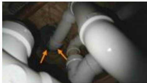
1st Floor Master Bathroom Shower Leaking At Drain
