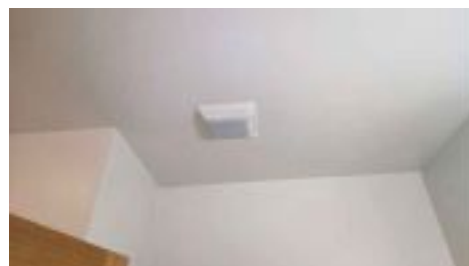
1st Floor Hall Bathroom Vent Light
