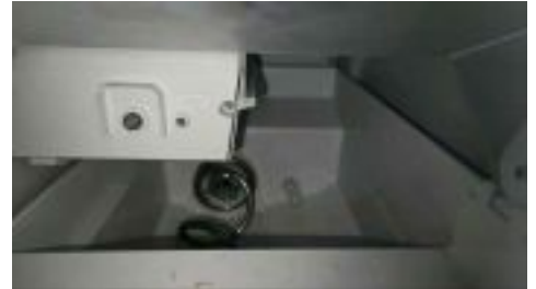
1st Floor Kitchen Refrigerator Ice Maker is Off
