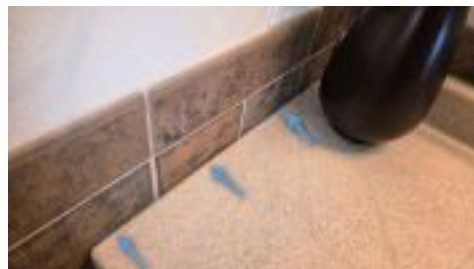
1st Floor Master Bathroom Sink Missing Caulking
