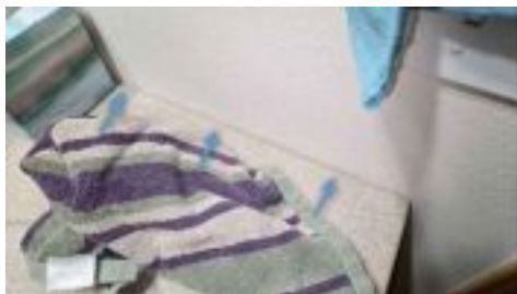
1st Floor Hall Bathroom Sink Missing Caulking
