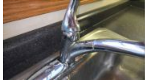
1st Floor Kitchen Cold Side Leaks Only When Operation
