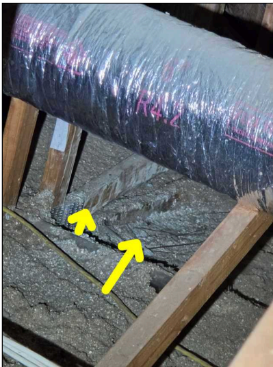
Evidence of moisture intrusion
