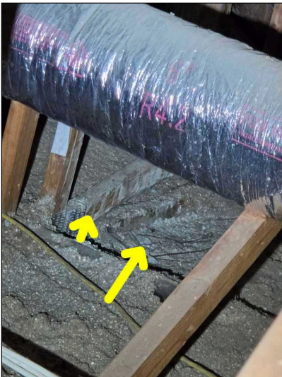
Evidence of moisture intrusion
