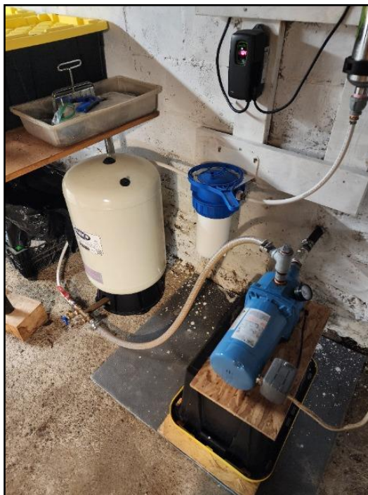
26. Well pump & pressure tank
