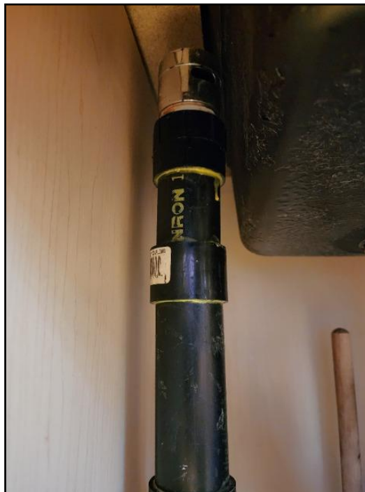
35. Automatic air vents
