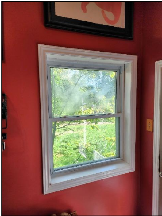
37. Lost seal on double glazing
