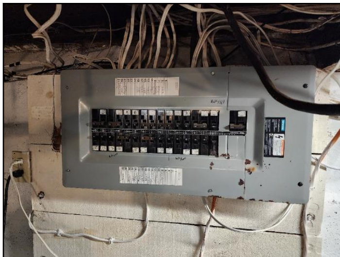
14. Main electrical disconnect
