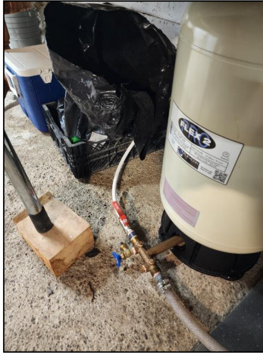
27. Main water shut off
