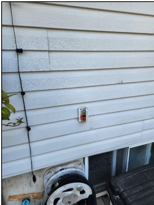
18. No GFCI/GFI (Ground Fault Circuit...
