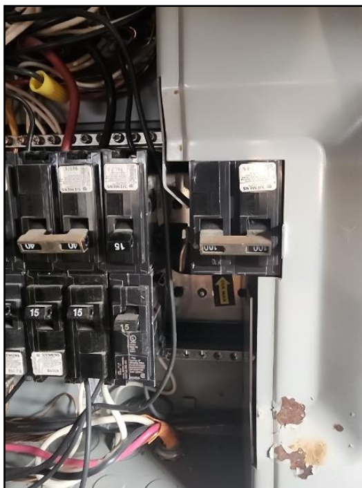
16. Wire crossing bus connections
