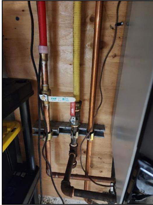
22. Main fuel shut off
