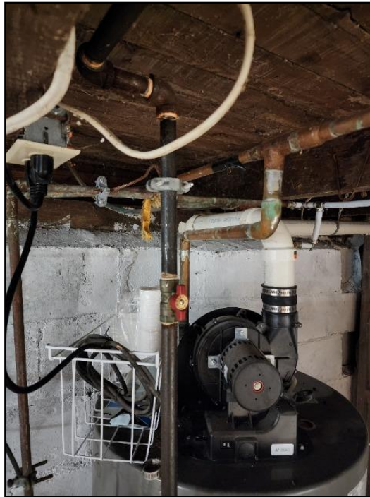
34. Main fuel shut off
