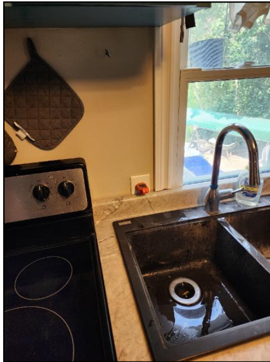
20. No GFCI/GFI (Ground Fault Circuit...
