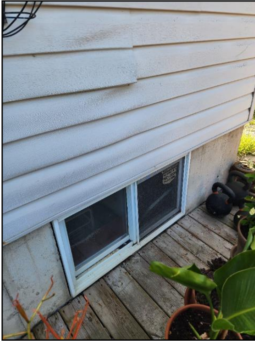
7. Caulking missing, incomplete or deteriorated
