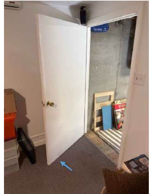
Basement Laundry Room Door Dragging On Carpet
