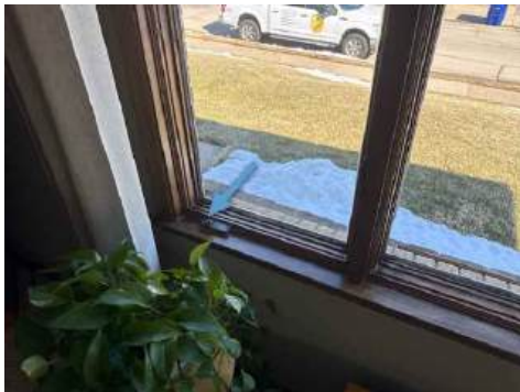
1st Floor Living Room Left Window Pane Missing Hand Crank
