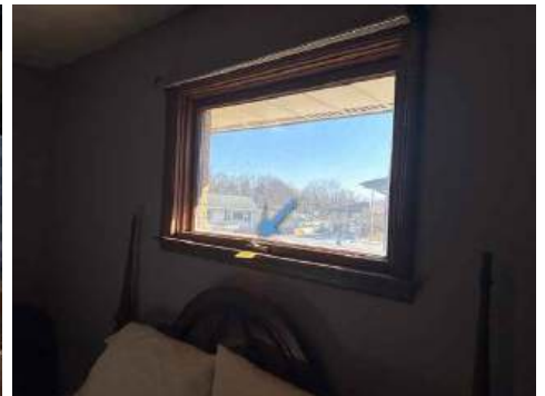
1st Floor Bedroom Window Missing Hand Crank
