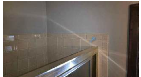
1st Floor Hall Bathroom Shower Enclosure Cracked
