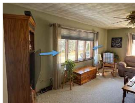
1st Floor Living Room Window Painted Shut From Outside
