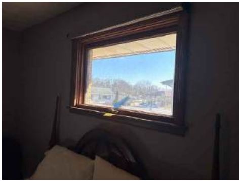
1st Floor Bedroom Window Unable To Test
