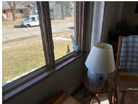
1st Floor Living Room Right Window Missing Hand Crank
