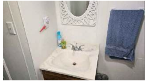
Basement Bathroom Outlet Loose
