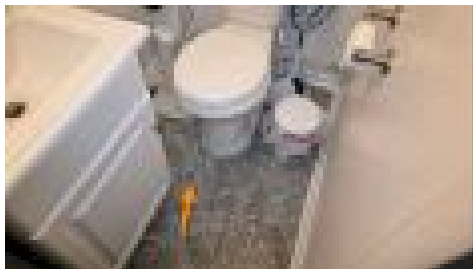
1st Floor Hall Bathroom By Toilet The Floor Sinks In
