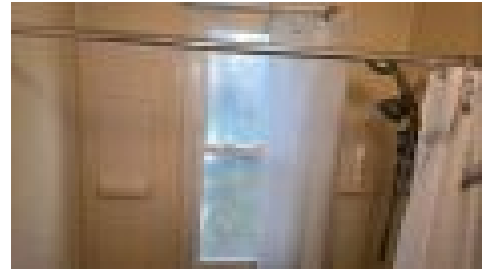
2nd Floor Hall Bathroom Window Will Just Drop
