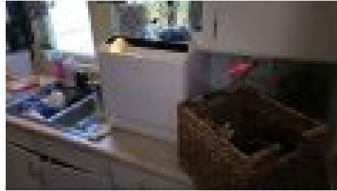
1st Floor Kitchen Outlet No GFCI Protection
