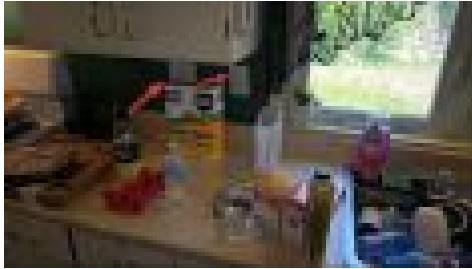
1st Floor Kitchen Outlets No GFCI Protections
