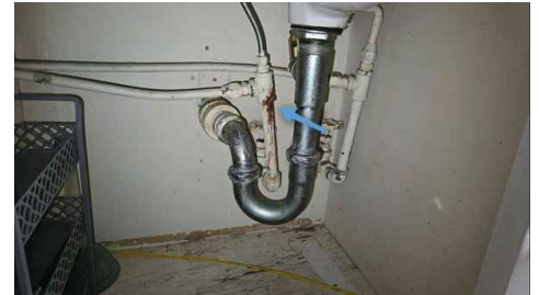
1st Floor Hall Bathroom Right Sink Corrosion On Supply
