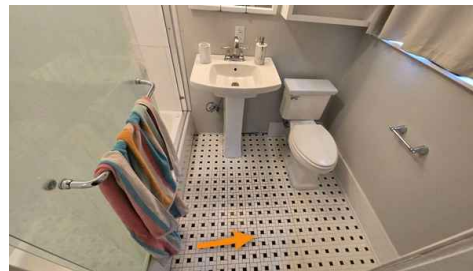
2nd Floor Master Bathroom Floor Dips Here
