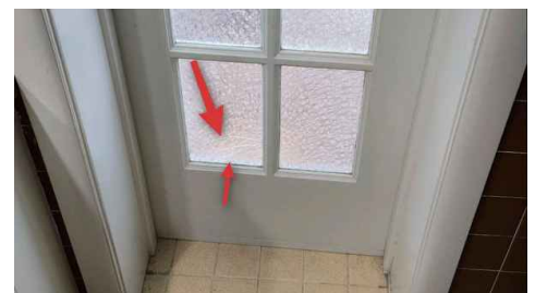
2nd Floor Hall Bathroom Door
