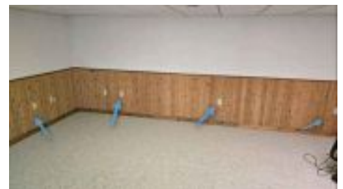
Basement Livingroom Outlets Open Ground
