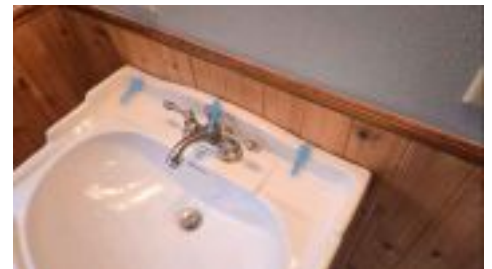
Basement Bathroom Sink Missing Caulking
